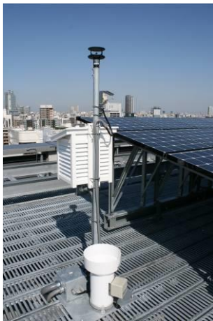
Figure 7 Picture of roof-top weather station used to measure ambient conditions used in the control system.
