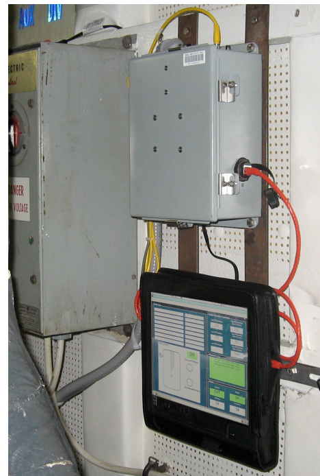
Fig. 5. NILM system as installed next to a power distribution panel on the USCGC ESCANABA. The NEMOmetrics sensor and data acquisition box, top, connects via Ethernet to a tablet PC, bottom.
