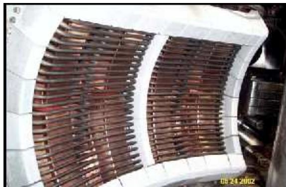
Figure 3-4: Picture of J-Antenna as installed in the vacuum vessel.
