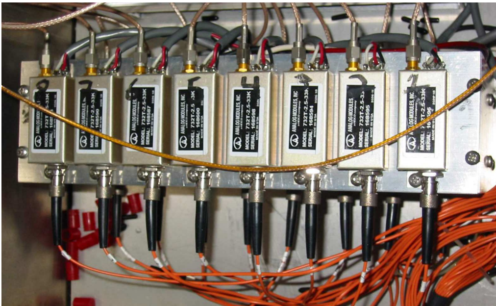
Figure 3-10: Top Shelf of the Fiber Optic Link Transmitters
