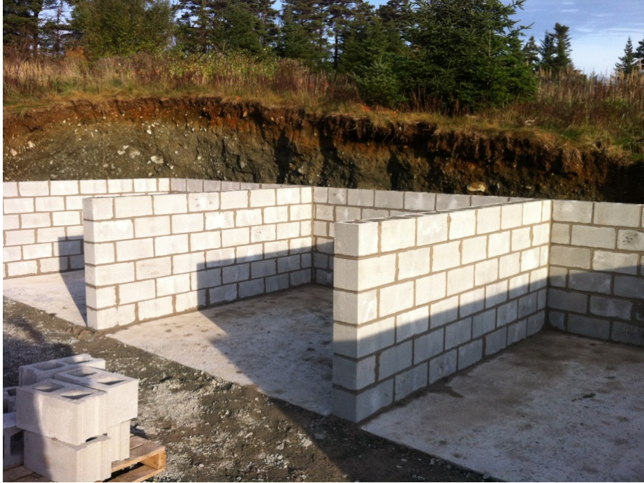
#3 - Finished collection bins of the compost platform
