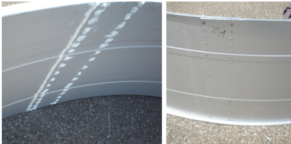
Figure 3.24 The wall sheet sections were overlapped approximately 10 cm. After sealant was applied they were connected with pop rivets.
