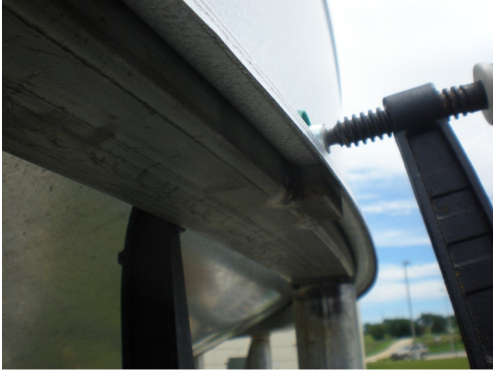
Figure 3.29 Self-tapping screws were used to attach the bottom ring of the silo to the hopper cone base.
