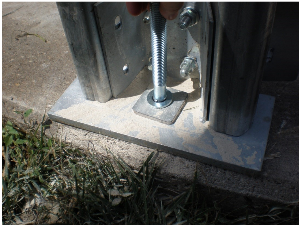
Figure 3.18 Anchor bolt securing a support leg of the SCAFCO hopper silo to the concrete pad.
