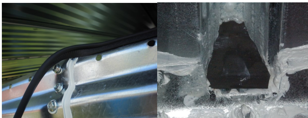
Figure 4.2. Rubber gasket attached between roof and edge of top wall sheet (left), and closed-cell foam block closing large gap at the end of the roof rib (right).
