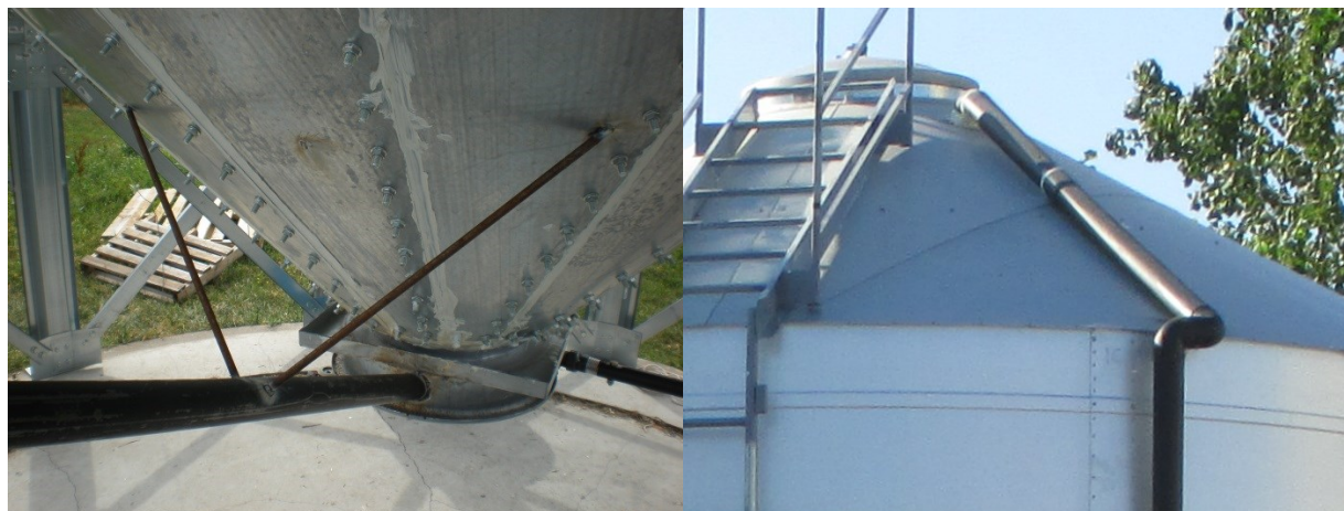
Figure 4.3. Showing the ThermoSiphon recirculation pipe connecting the \text{PH}_3 reaction chamber below the hopper (left) and the headspace (right).
