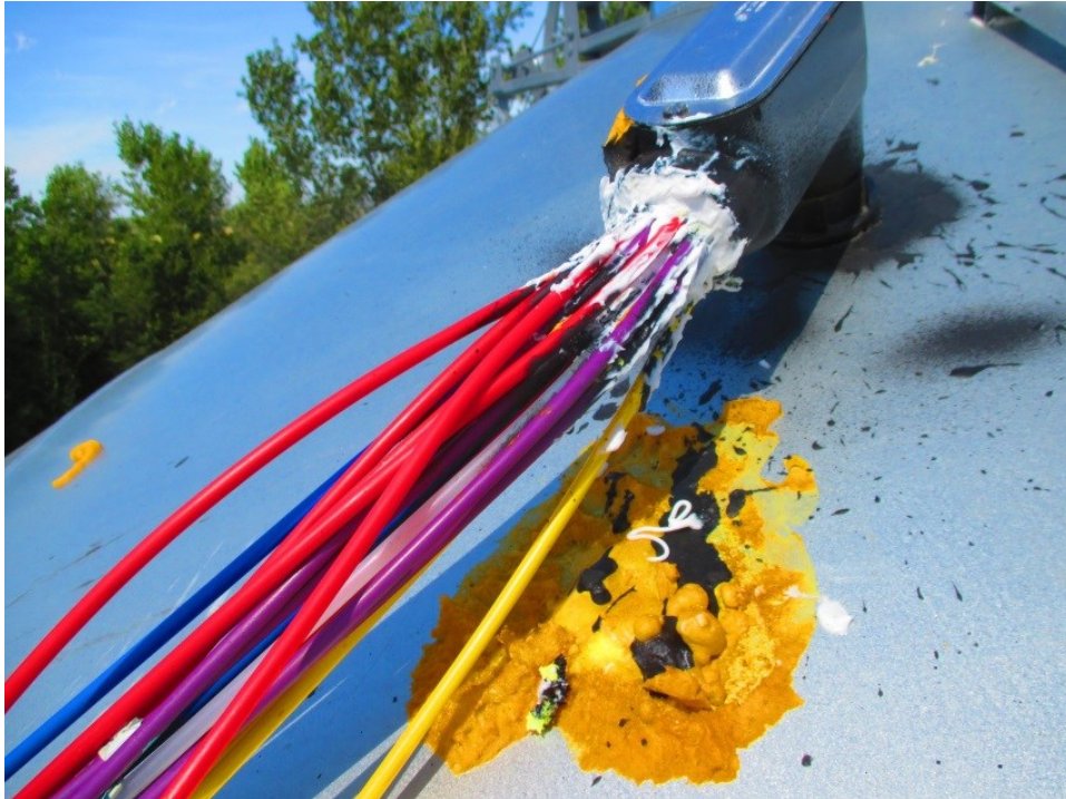
Figure 4.7. Monitoring lines exiting silo roof. The fitting was filled with closed-cell expanding foam and sealed with silicone caulk around the lines.
