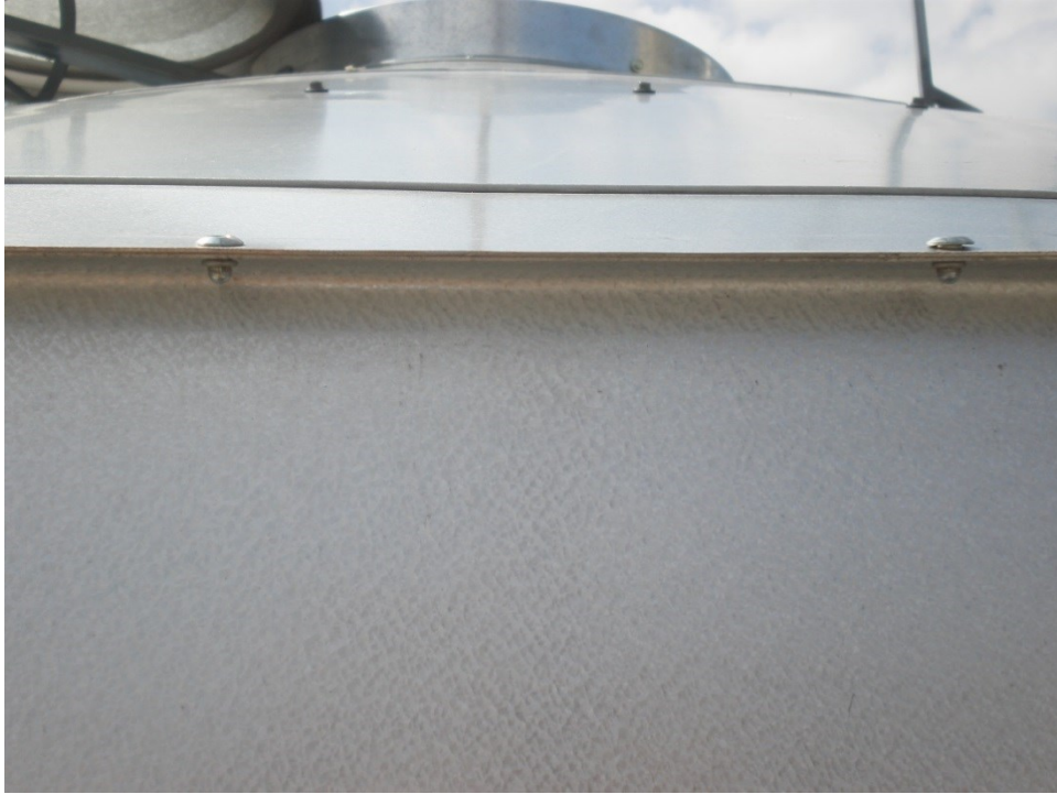
Figure 3.25 The roof section was lifted onto the top wall ring and attached with pop rivets.
