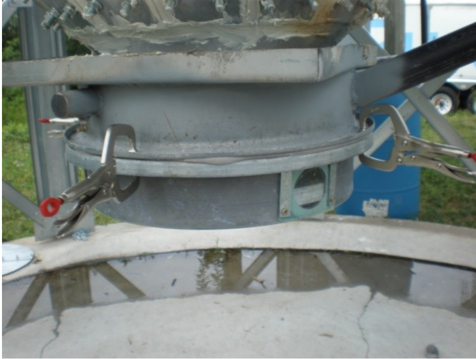
Figure 4.4. Airtight \text{PH}_3 reaction chamber installed on the underside of the hopper bottom.
