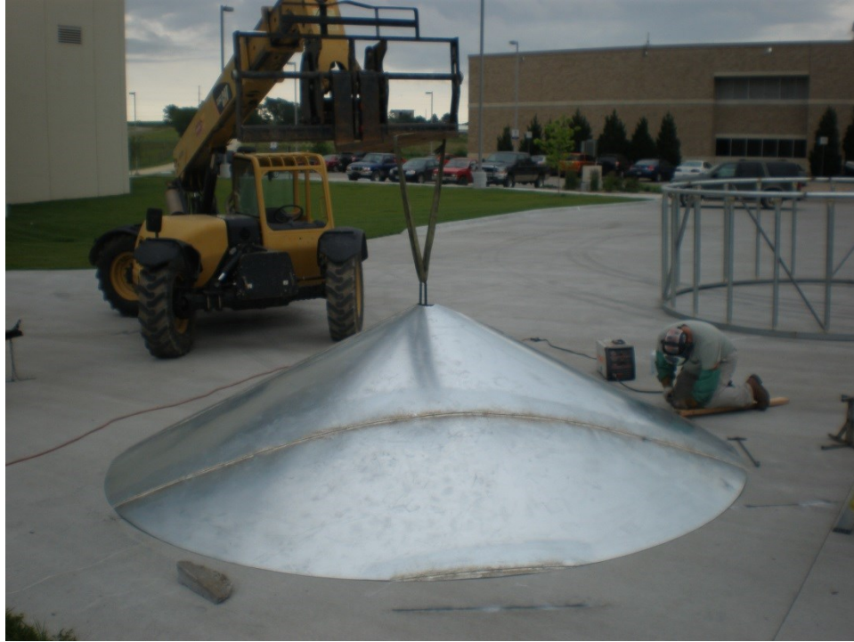
Figure 3.22 Lifting of the roof sheet of the Bird's silo and forming it into the shape of a cone before welding the final seam.
