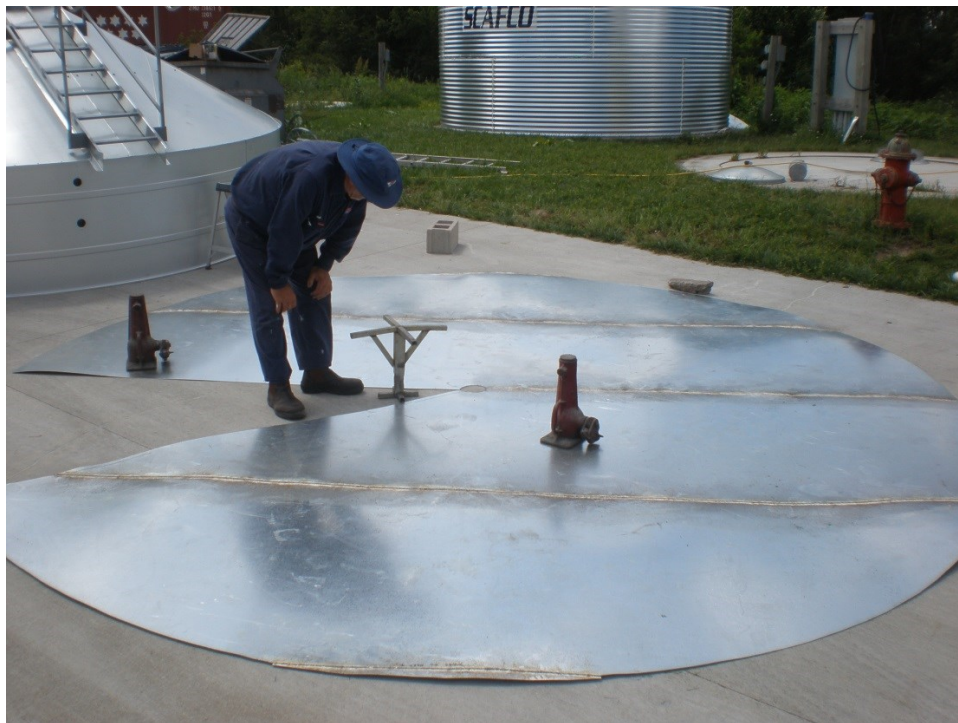
Figure 3.21 Inspecting the welded hopper sections before forming the sheet into a cone and welding it to the base structure.
