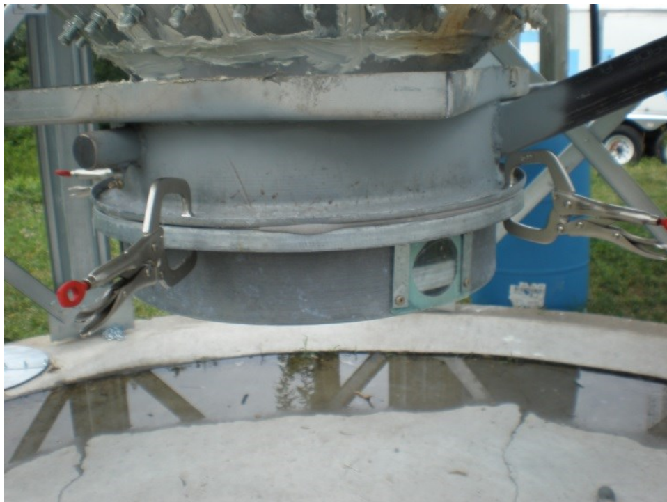
Figure 3.32 Phosphine reaction chamber installed below the butterfly valve of the hopper bottom silo.
