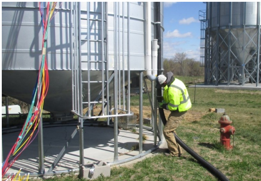
Figure 4.9. Attaching the VAPORPH 3 OS® to the ThermoSiphon. The gas was directed to the headspace using a valve on the ThermoSiphon.
