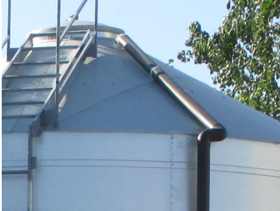
Figure 3.34 Thermosiphon piping extending along the south roof panel and connecting into the headspace of the Bird's silo.
