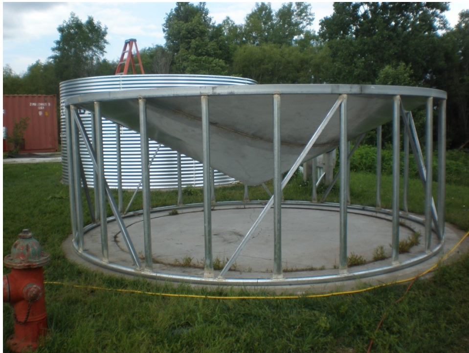
Figure 3.28 The preassembled hopper cone was placed inside the base support structure and welded to it.
