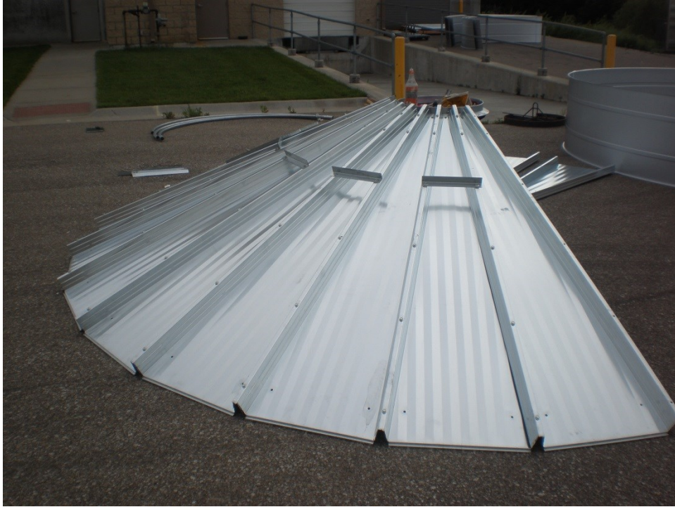
Figure 3.6 A-shaped sections with overlapping ribs formed the roof of the SCAFCO silo.
