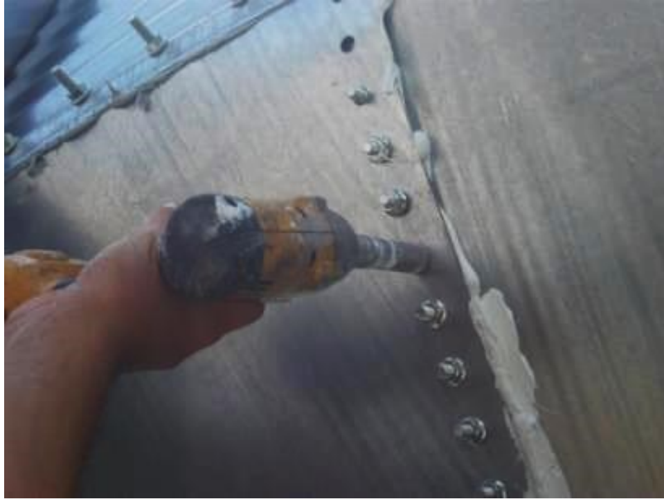
Figure 3.20 Tightening the bolts on the hopper after application of polyurethane sealant into the gap between sheets.
