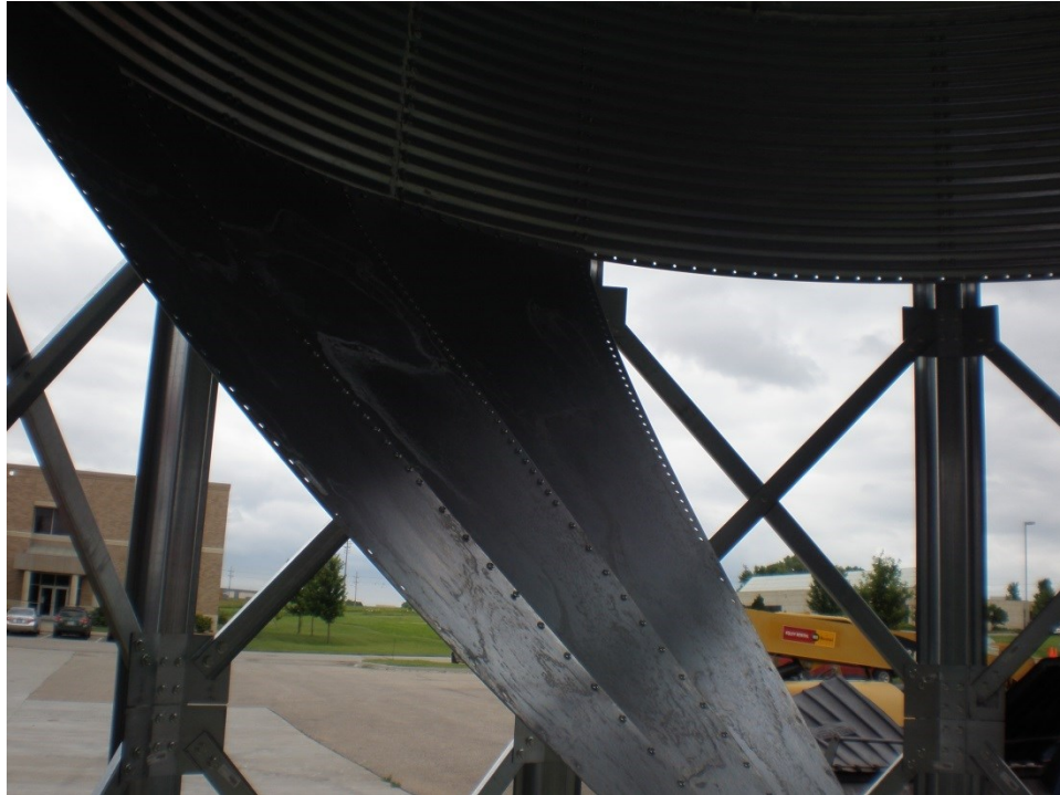
Figure 3.19 All of the hopper sheets were put in place before applying sealant between the sheets and tightening the bolts.
