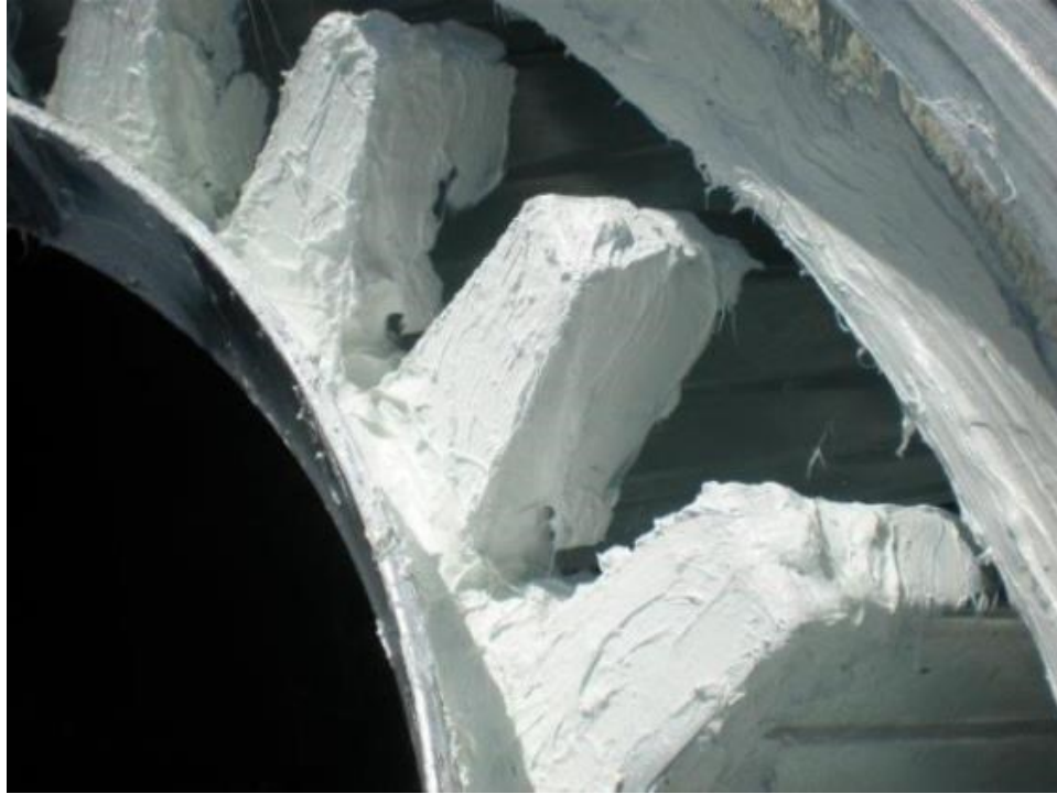
Figure 3.10 Metal flashing pieces on the ends of the roof rib openings after covering with sealant.
