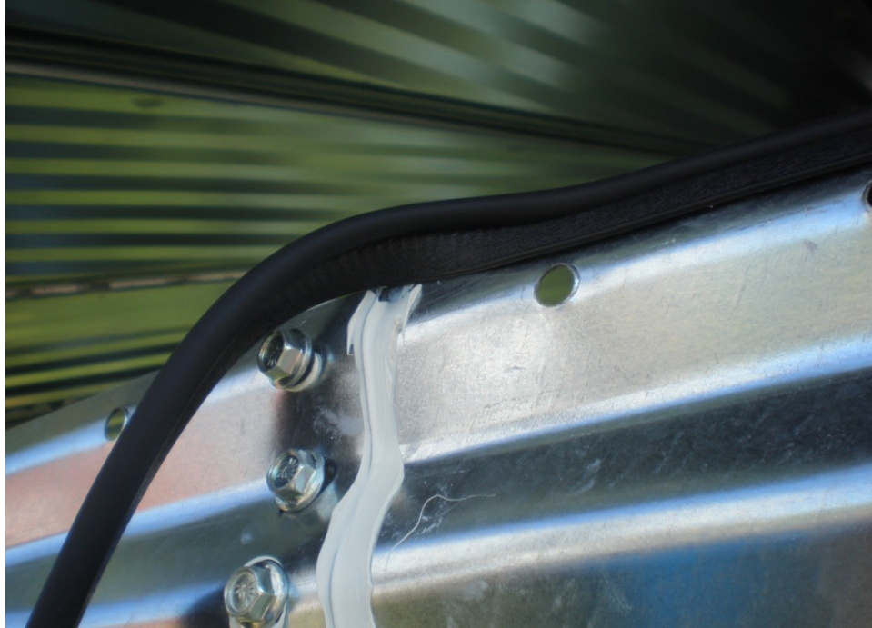
Figure 3.16 Rubber gasket that was installed around the entirety of the top wall sheets to help seal the seam between the top wall and roof panels.
