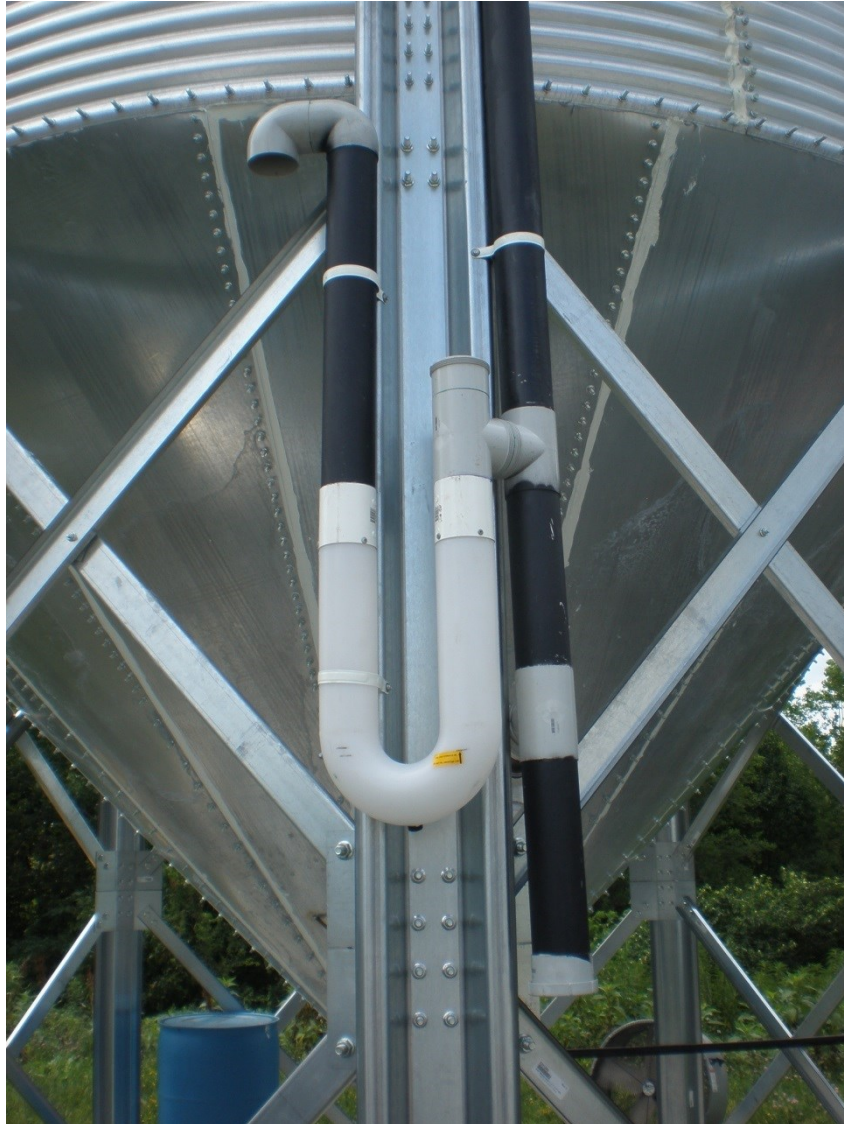
Figure 3.3 U-tube pressure relief valve piping connected near the bottom portion of the thermosiphon piping. Also used as a monitor for pressure testing of the sealed silos.
