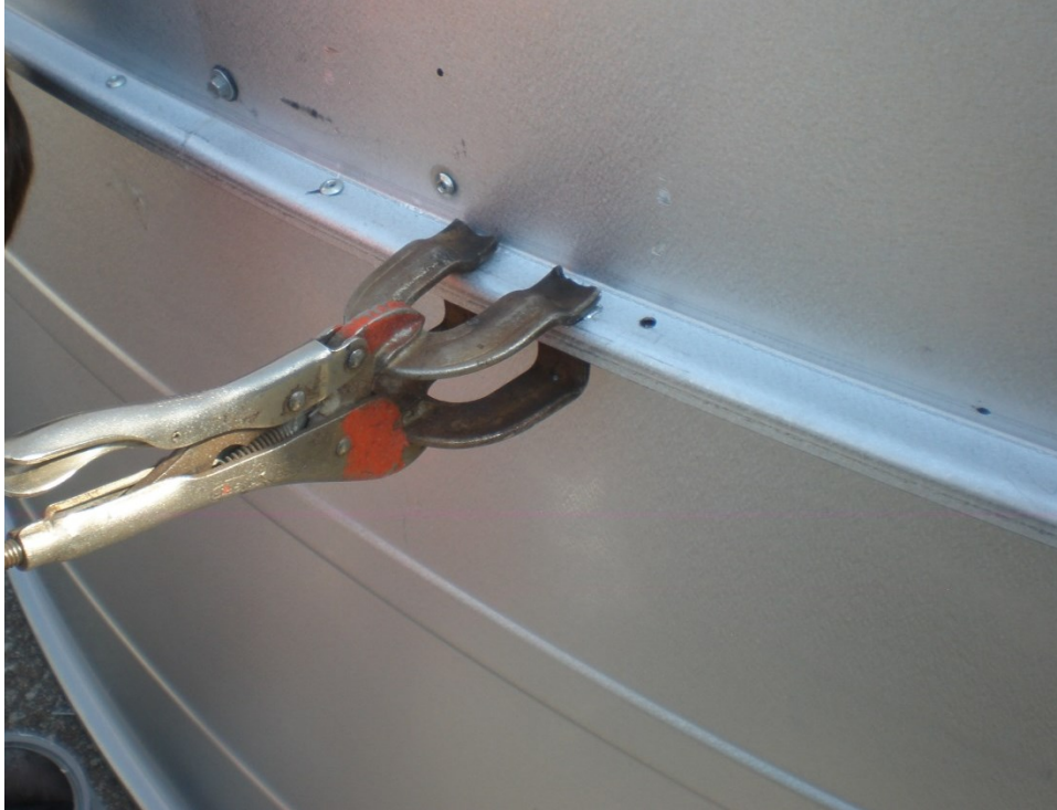
Figure 3.27 Close-up view of connecting the wall rings to each other using pop rivets.
