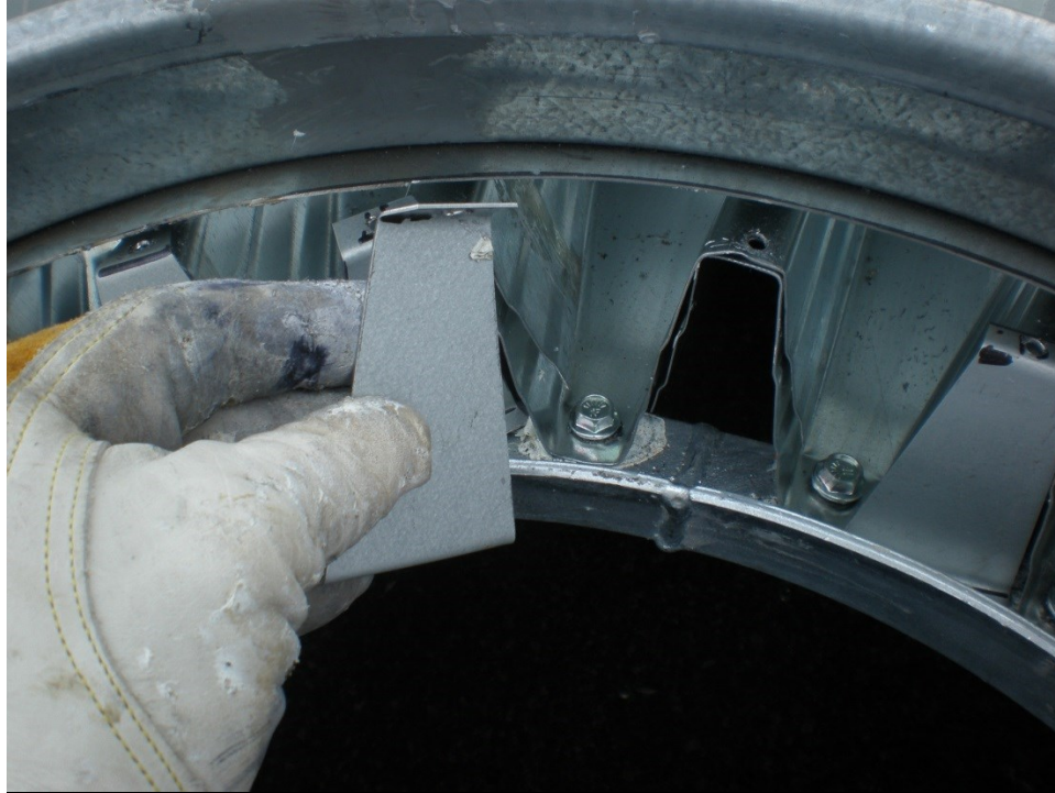
Figure 3.9 Metal flashing piece to be screwed onto the roof rib opening to cover the ends of the roof ribs.
