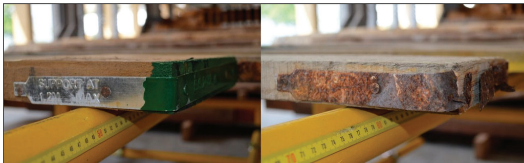
FIGURE 2. Illustration of an end band before and after exposure to oceanic atmosphere
