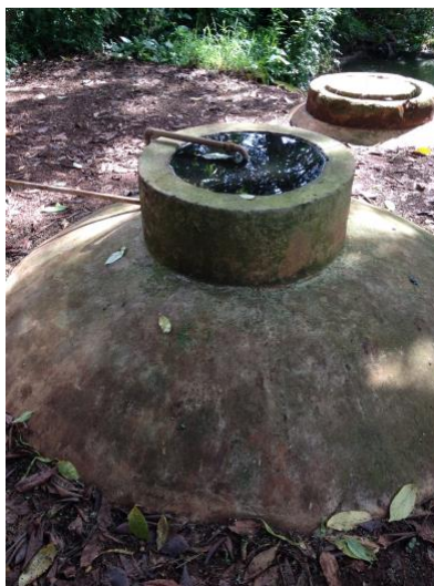
Figure A.5: Main digester and expansion chamber
