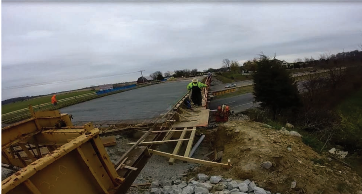
Figure 5.5 Picture of finalized internally cured high performance bridge deck on SR 46 over I-74.
