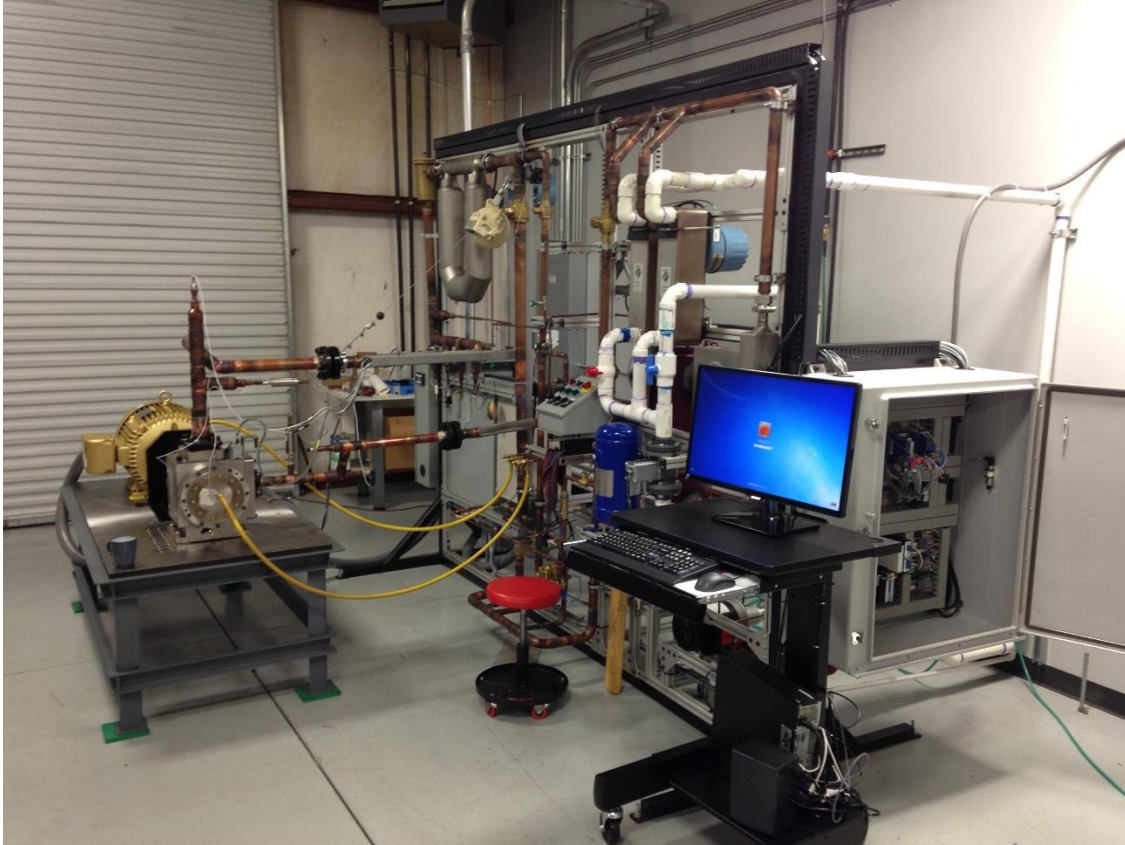
Figure 3: Photo of 141 kW hot gas bypass test stand
