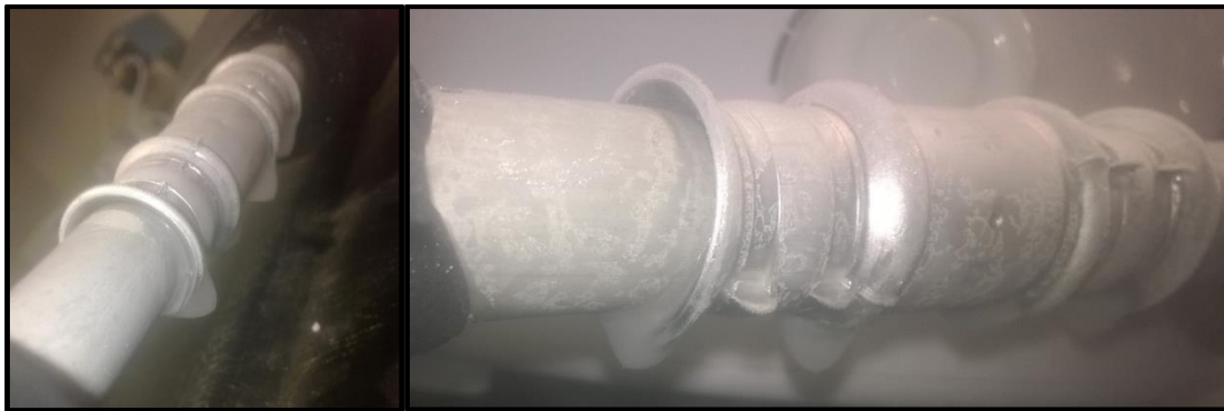
Figure 10: Ice formation at the joints of the fittings
