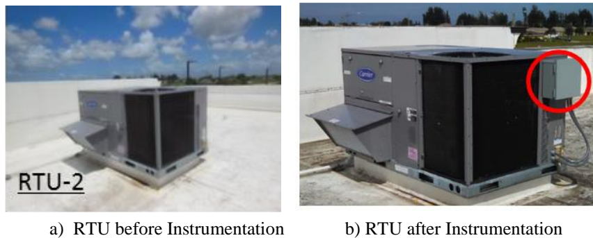
Figure 13 RTUs before and after Instrumentation
