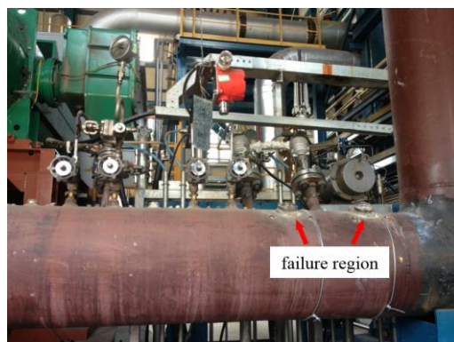
Figure 1: Fatigue fracture of the thermowells
