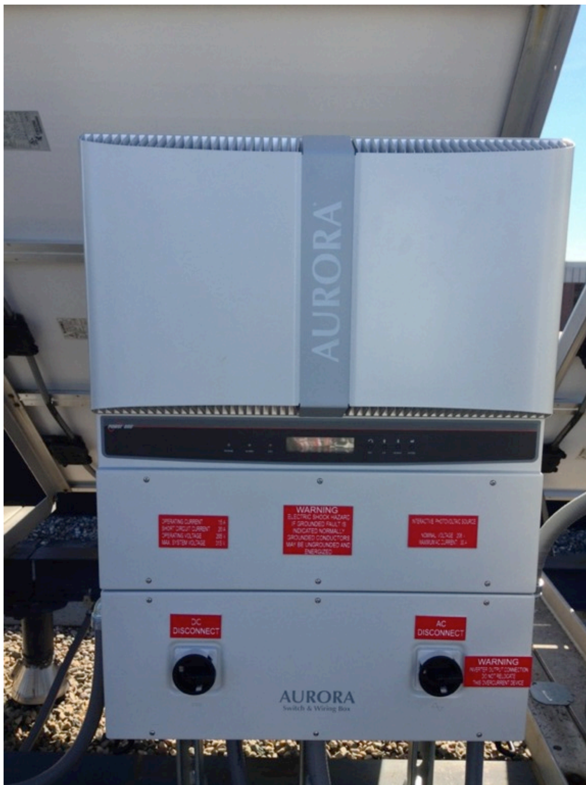
Figure C.7 Power-One PVI-10.0-I-OUTD-US 208V Inverter
