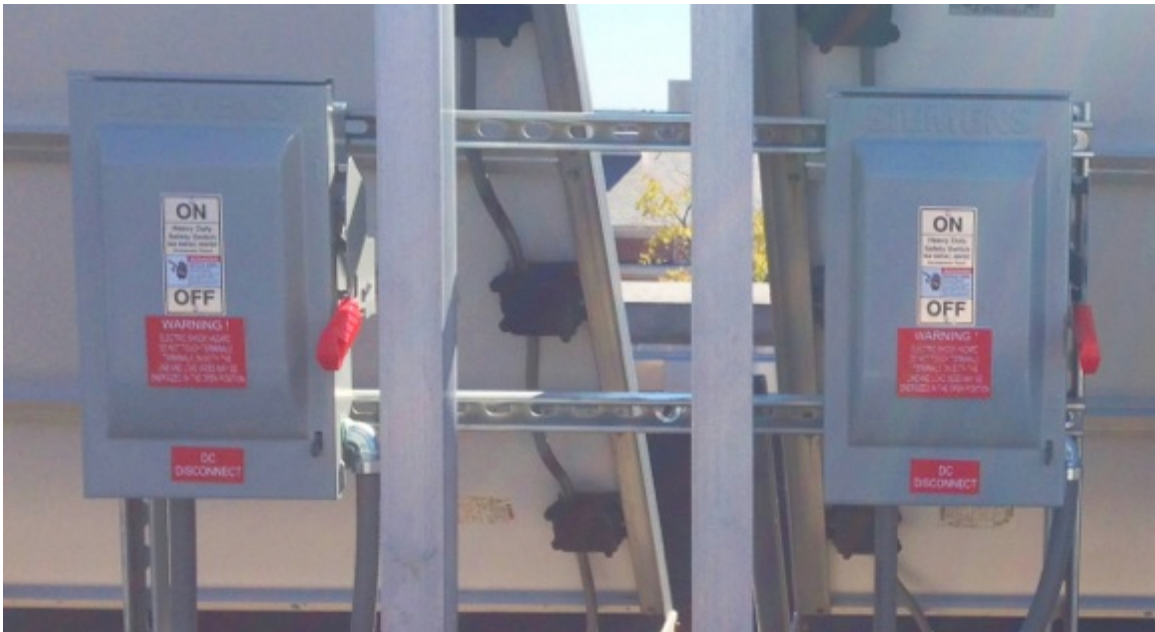
Figure C.6 Dual Siemens Heavy Duty 600VDC 60A Non-Fused DC Disconnects
