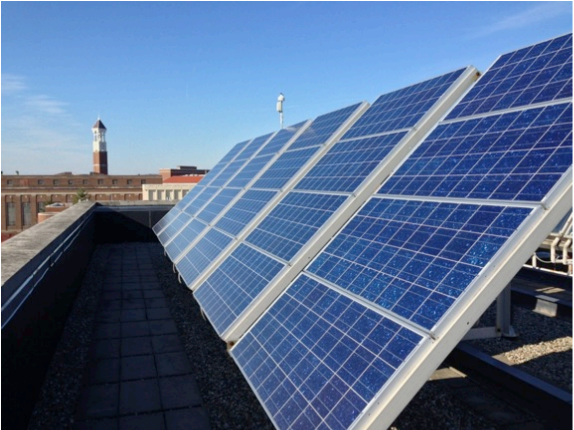
Figure C.4 3 kW Solar PV Array
