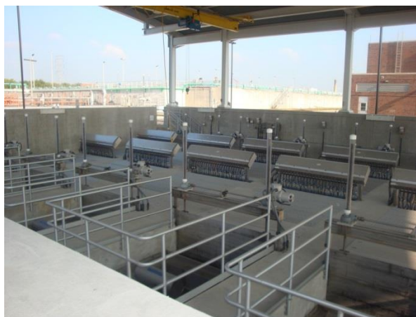
Figure 10. UV disinfection reactor at the Belmont WWTP
