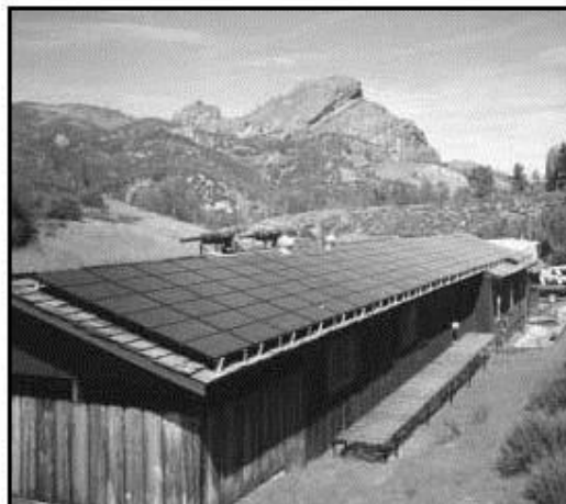
A PV system at the Pinnacles National Monument in California eliminates a $20,000 annual fuel bill for a diesel generator that produced each year 143 tons of carbon dioxide—a greenhouse gas.
