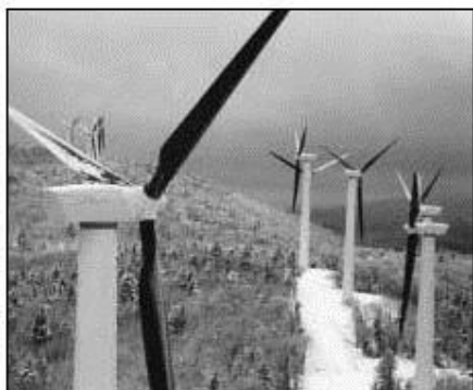
The 6-MW Green Mountain power plant in Searsburg, Vermont, consists of eleven 550-kW wind turbines.
