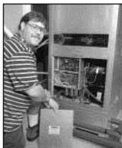
This homeowner in Aurora, Colorado, uses a GHP to heat and cool his home.
