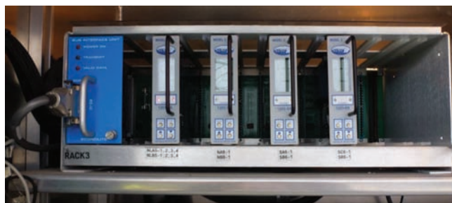
Figure 2.5 Detector bus interface unit (BIU) with approach, phase, and lane labeled.
