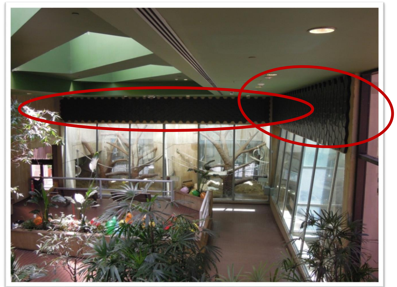
Installed microperforated panels in the Great Ape House of the Smithsonian National Zoo
