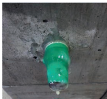
Figure 3. Insulated end of steel bar during corrosion.
