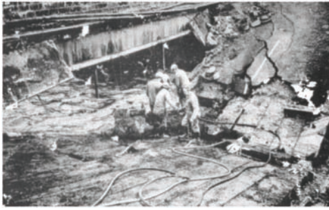
Figure 1. Collapse of Ynys-y-gwas Bridge in Port Talbot.
