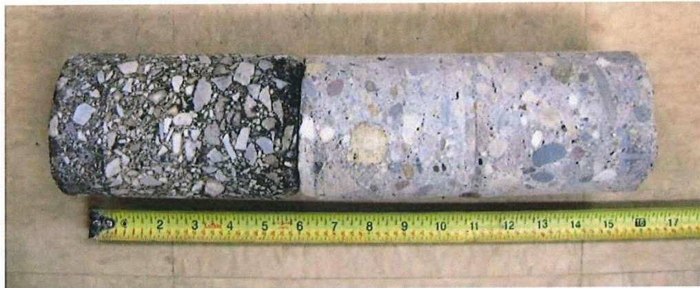
PC_S2-RB-11 – Station 18+00, Line “I65”, SB Slow Lane
