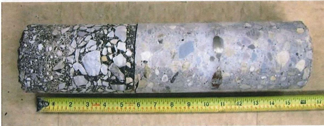
PC_S2-RB-59 – Station 114+00, Line “I65”, SB Slow Lane
