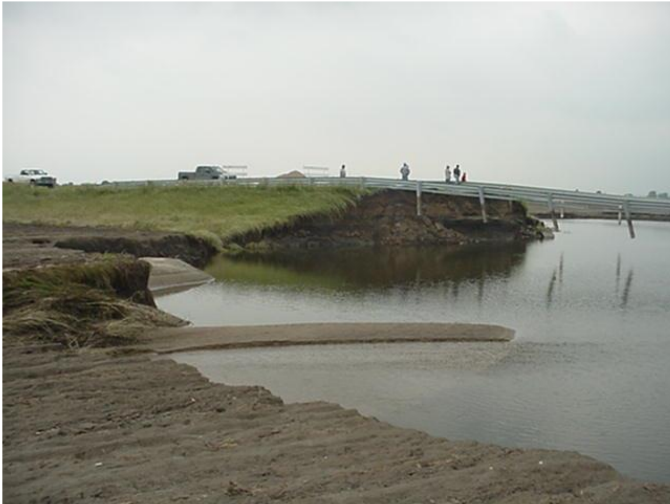
2008 site photo, structure damage & scour
