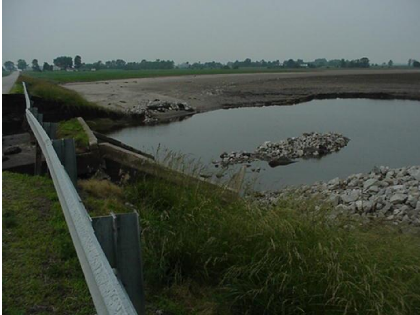
2008 site photo, outlet and scour hole
