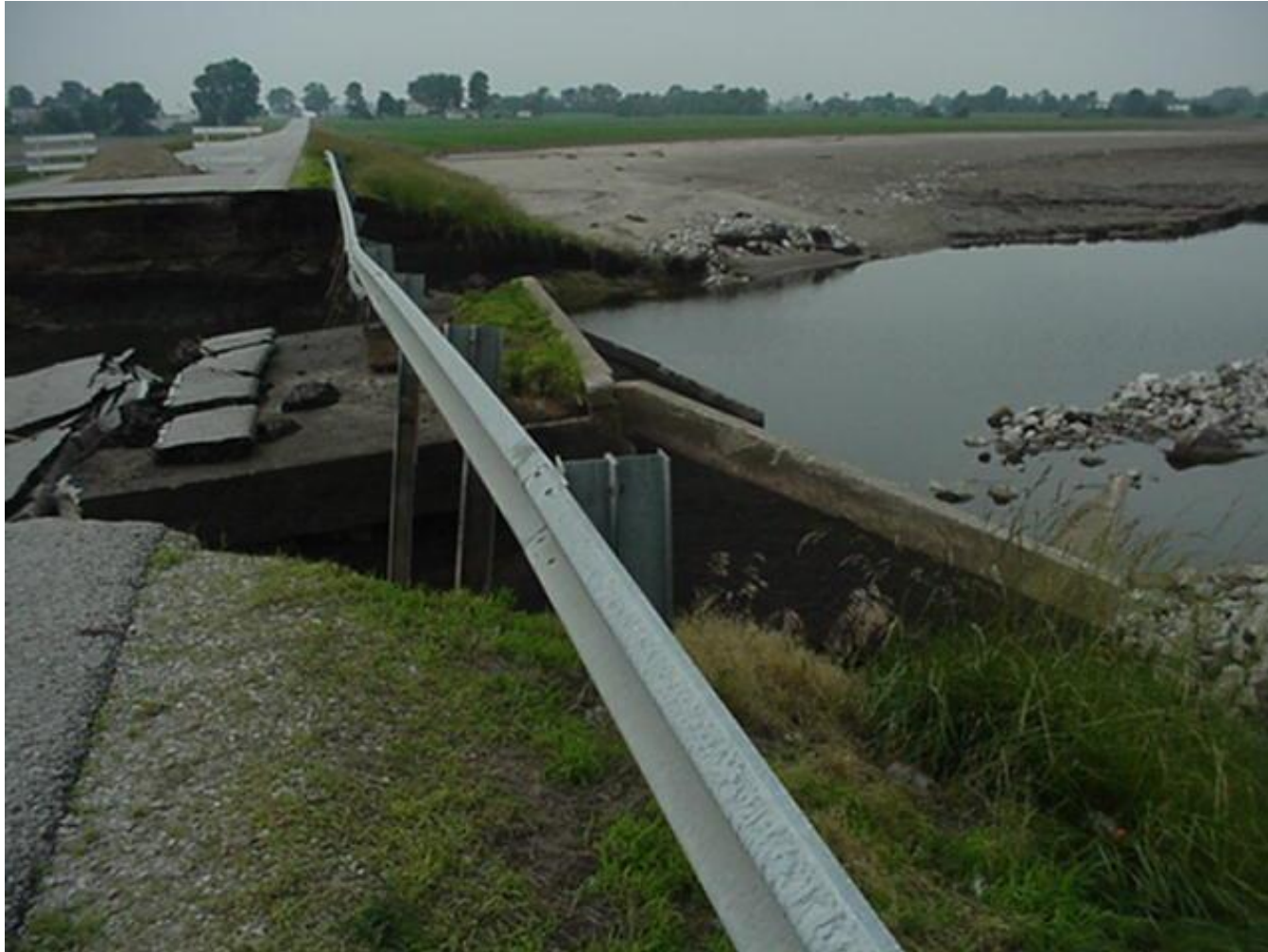
2008 site photo, outlet and scour hole
