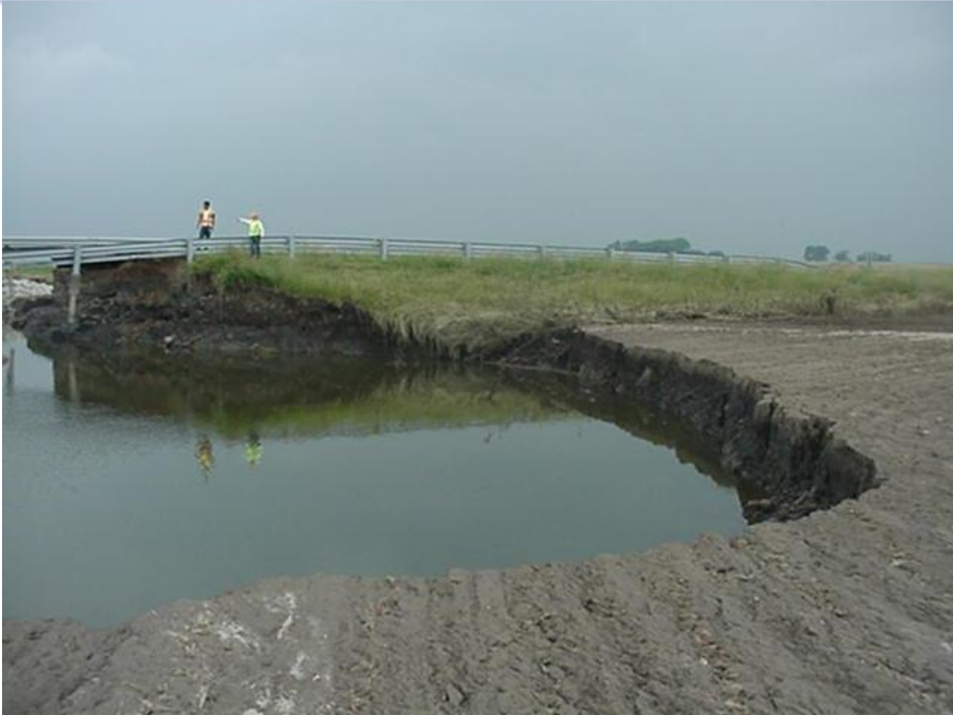
2008 site photo, structure damage & scour
