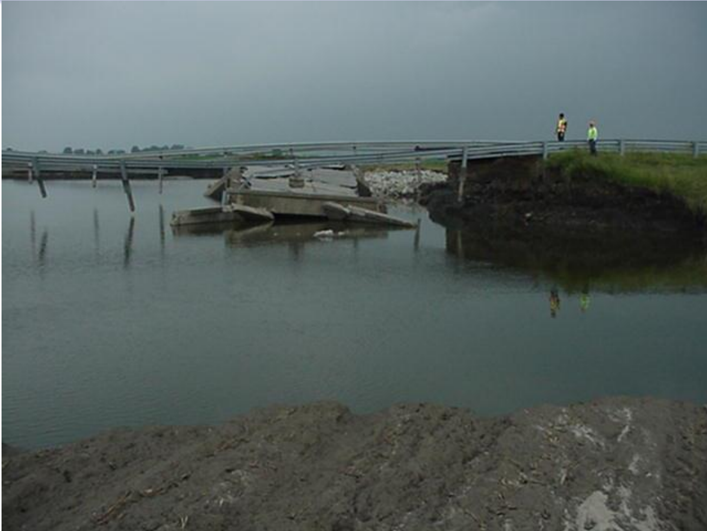
2008 site photo, structure damage & scour
