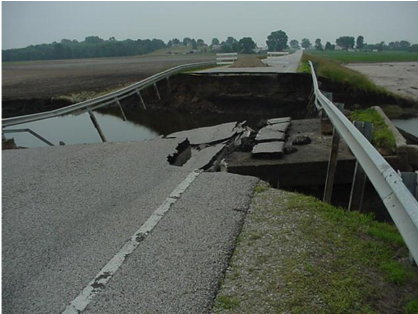
2008 site photo, structure & road damage
