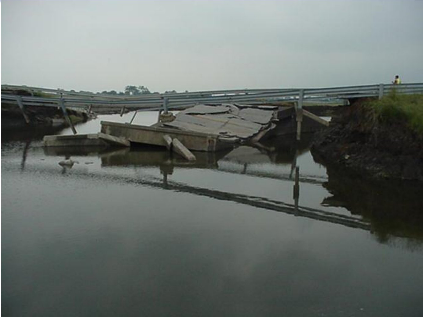
2008 site photo, structure damage
