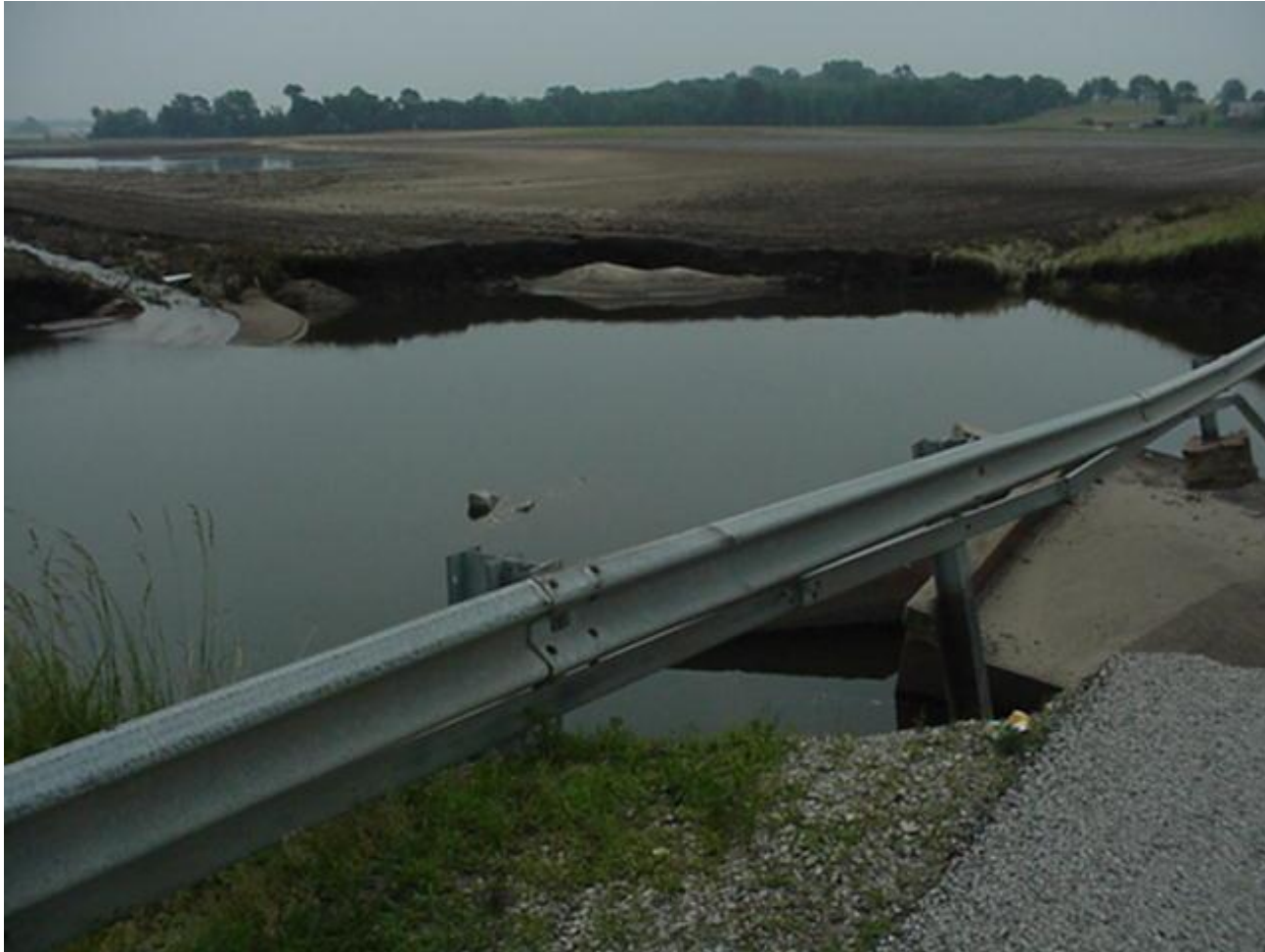
2008 site photo, contraction scour
