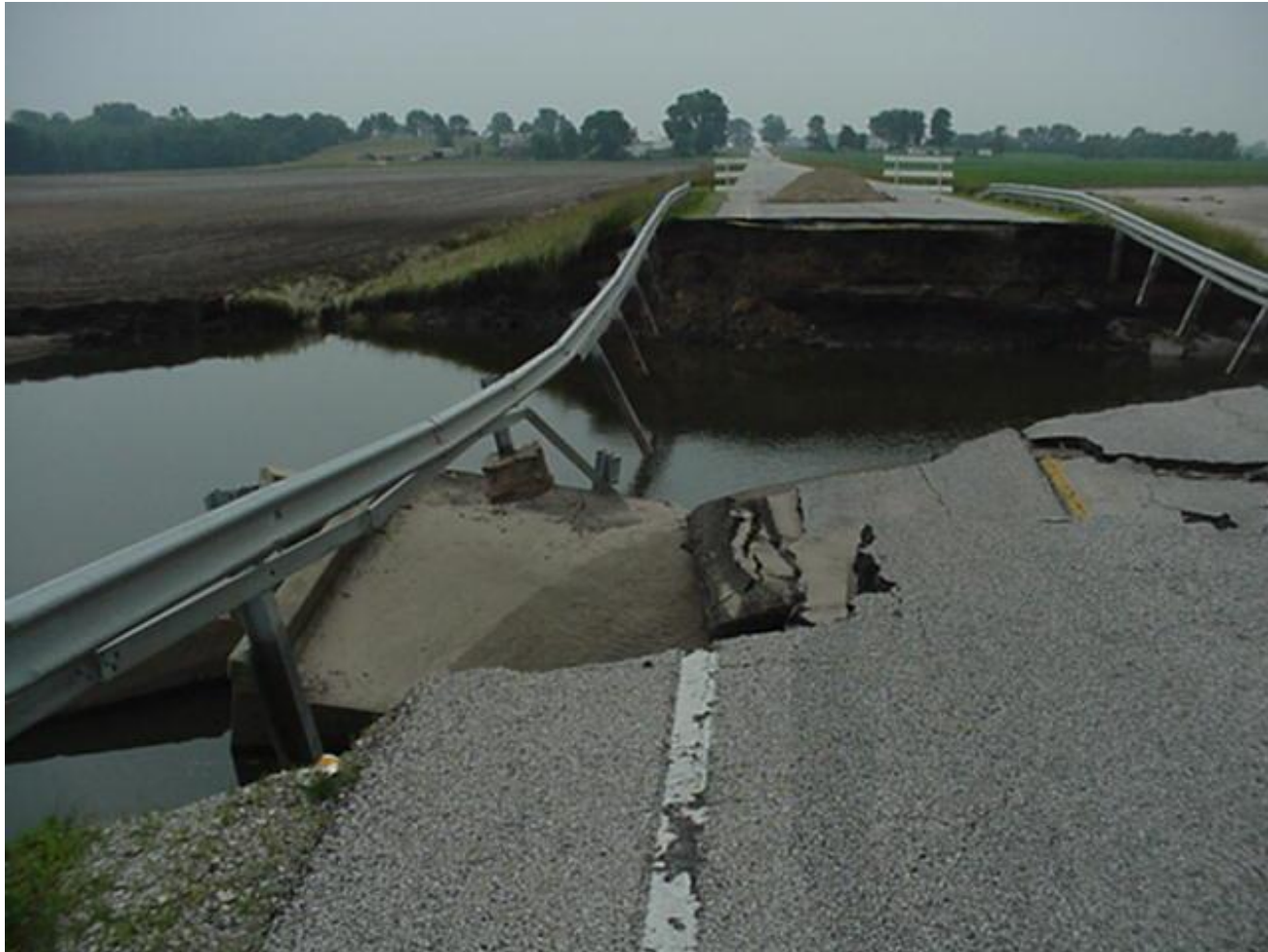
2008 site photo, structure damage
