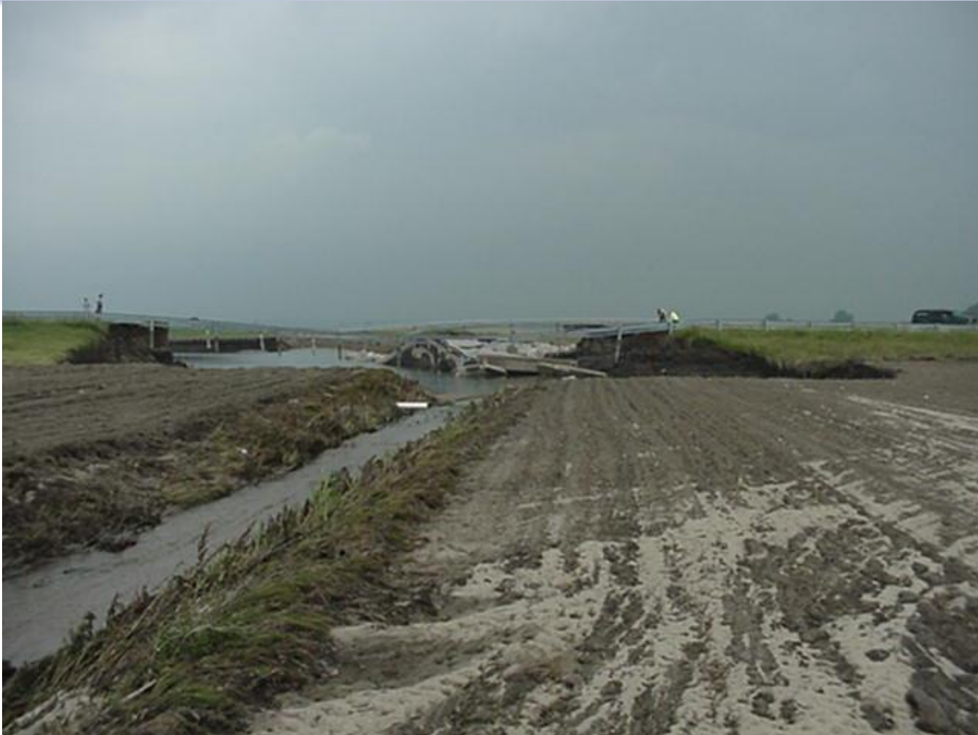
2008 site photo, structure damage & scour
