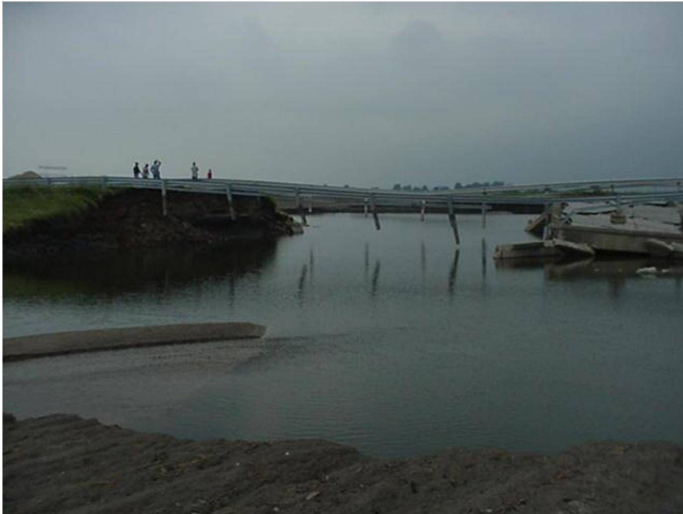
2008 site photo, structure damage & scour
