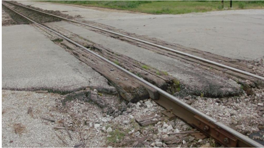
Timber and Asphalt – Poor Condition
