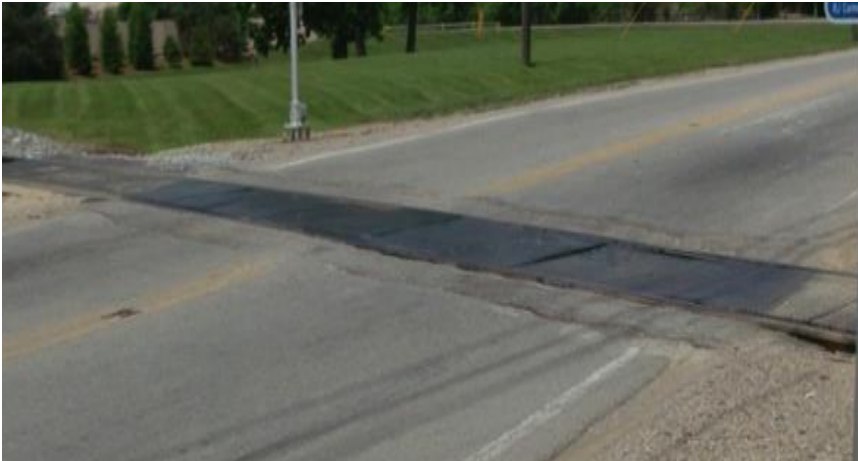
Full-Depth Rubber – Poor Condition
