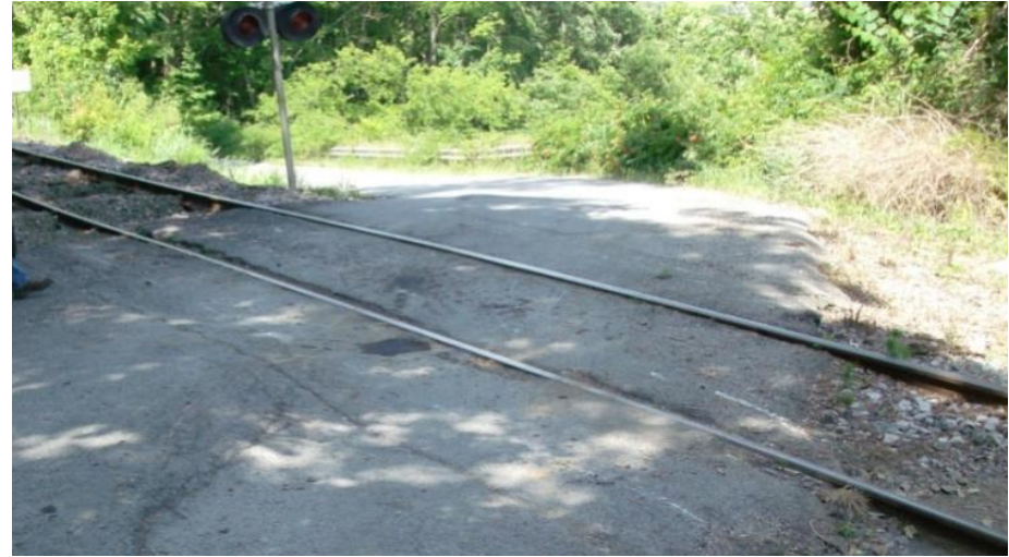
All-Asphalt – Poor Condition
