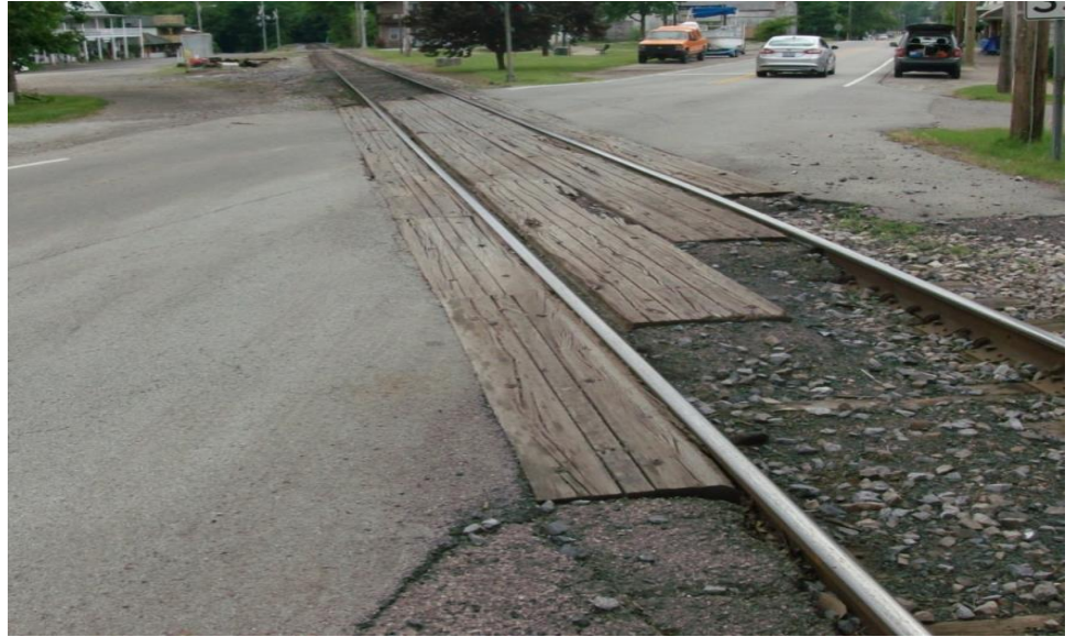
All Timber – Poor Condition
