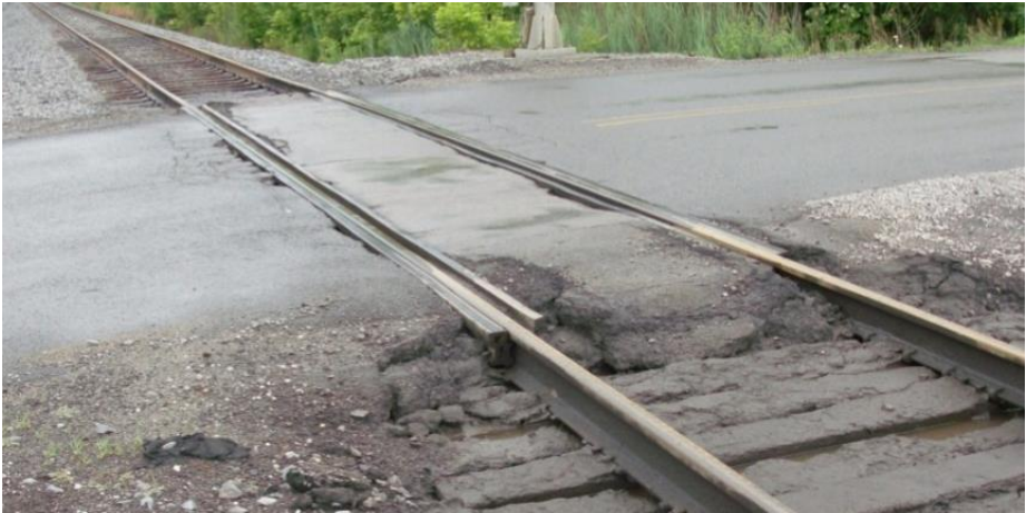
Rubber Seal and Asphalt – Poor Condition
