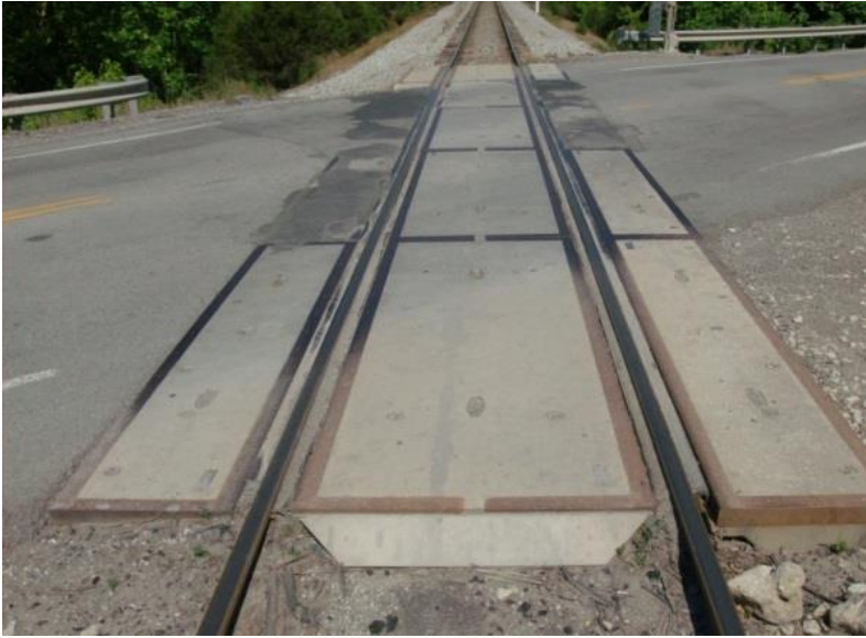
Concrete Panel – Poor Condition
