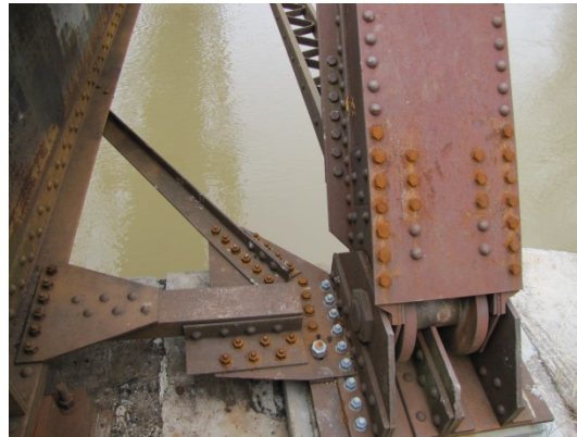
Replaced steel rivets with H.S. bolts - Deterioration
