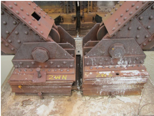
Steel shims installed below bearings – Pier Settlement
