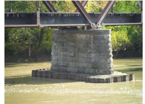
Installed steel channel walers – Erosion and Undermining
