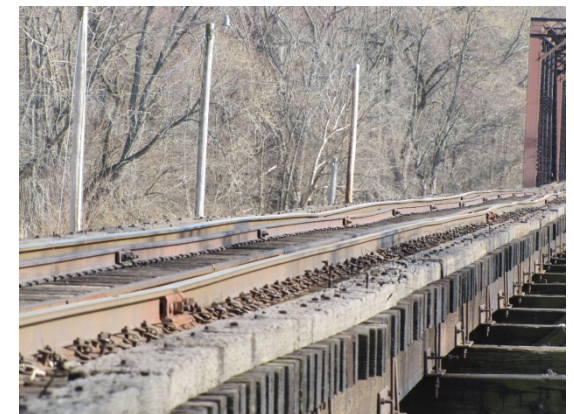
Maintain track alignment Settlement & Deterioration
