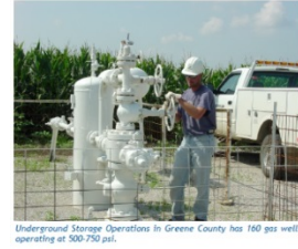
Underground Storage Operations in Greene County has 160 gas wells operating at 500-750 psi.
