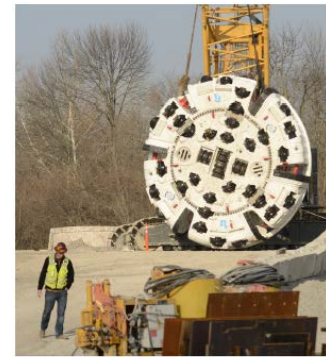
A tunnel boring machine with a 20-foot diameter cutter head is now drilling the Deep Rock Tunnel Connector, the first segment of the 25-mile Indianapolis Tunnel System that will capture combined sewer overflows.
