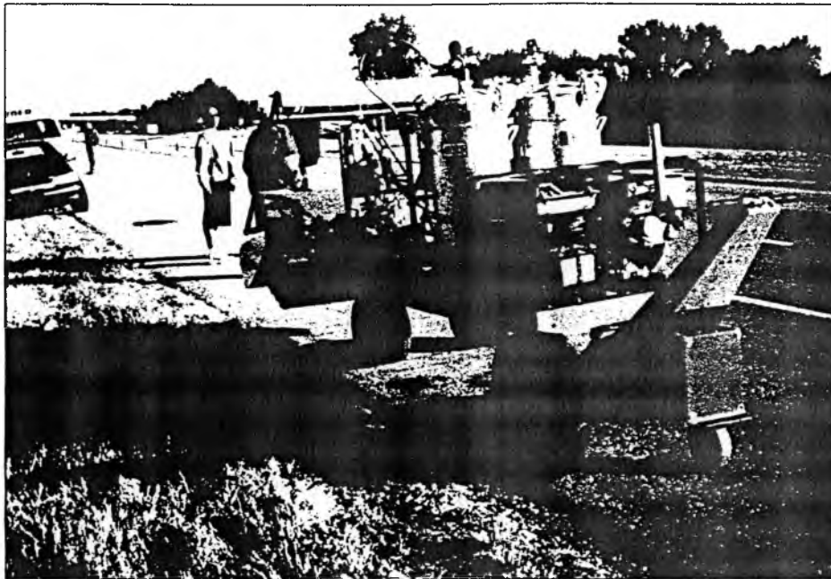
Convergent Spray Technology is applied in 4 hours as an anti-skid overlay on a bridge deck on Interstate 65 south of Huntsville.
