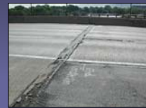
Deteriorated Pavement Joints
