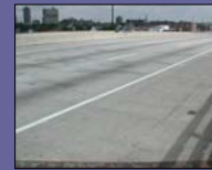
Deteriorated Bridge Decks
