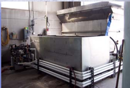
WDM Brine Production Unit
