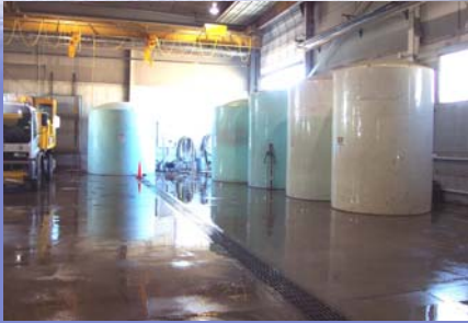
Brine Storage Tanks
