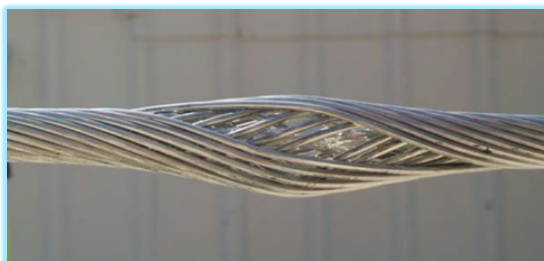
Figure 13 - Extreme example of conductor birdcaging by uncoiling/deformation of the outer aluminum conductor wire strands
