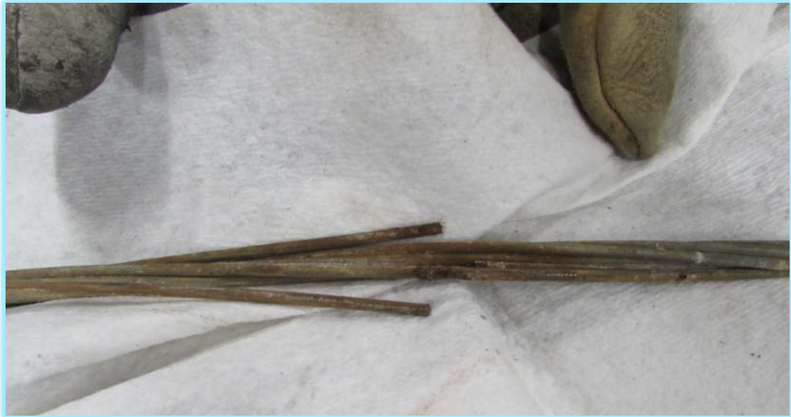
Figure 9 – ACSR/SD broken steel strands due to localized corrosion
