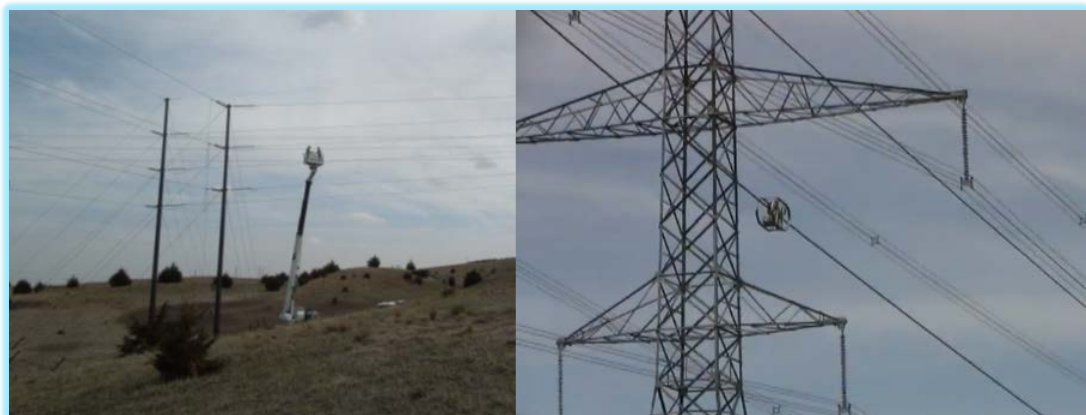
Figure 29 – Transmission line electromagnetic testing
