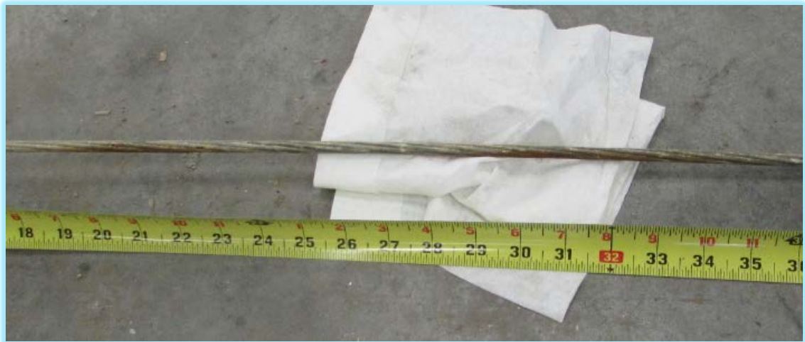
Figure 7 – Steel wire corrosion with the galvanization layer attacked in 8 to 10 inch intervals
