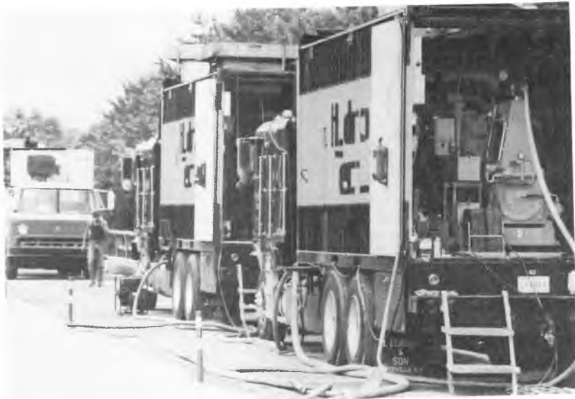
Each nozzle for hydrodemolition requires a truck containing a high pressure pump to provide 35 gpm at 17,000 psi.
