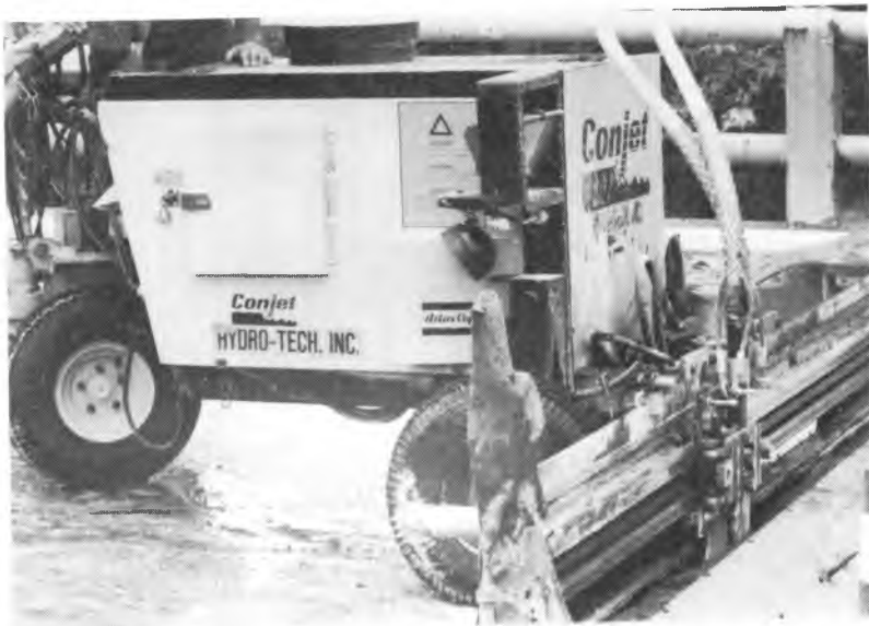
The slave used to remove concrete has two nozzles that connect to a high pressure pump and move along the front of the slave.
