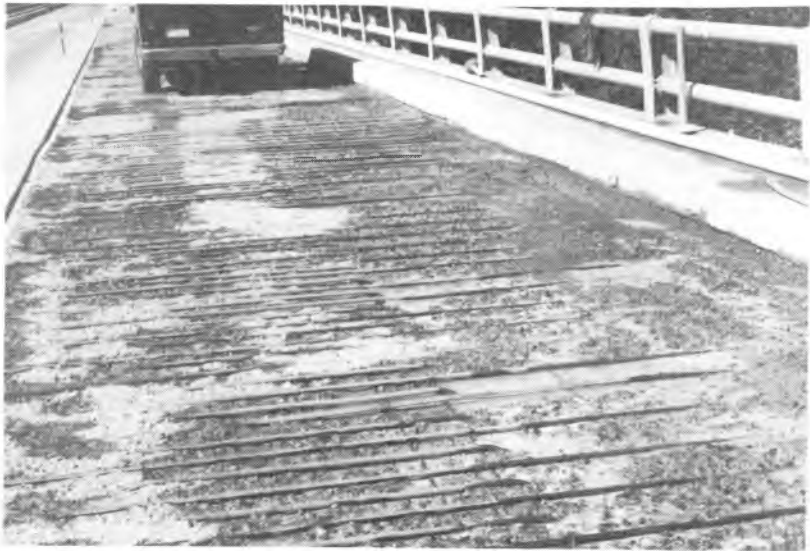
The finish section is ready for final cleaning; note excellent surface for bonding and clean re-steel.
