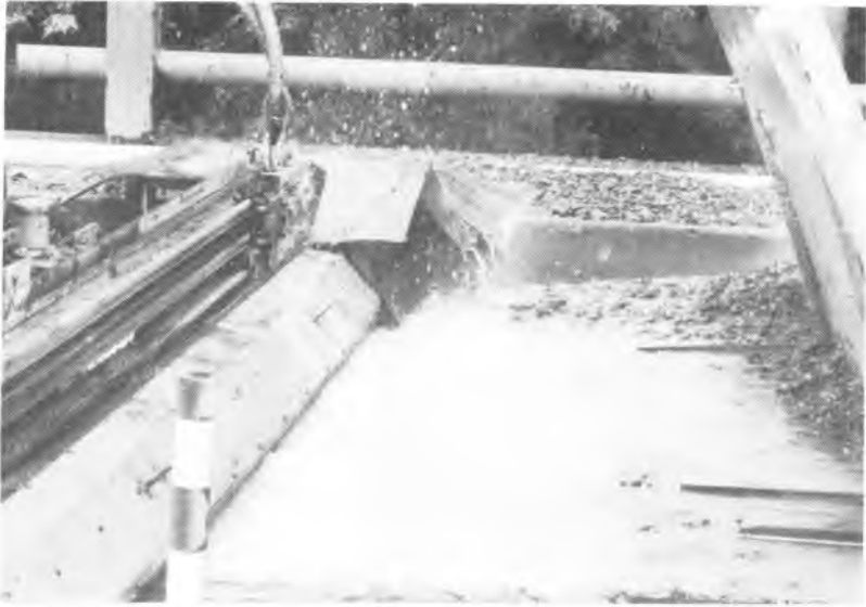
The slave is in action next to curb with protectors to keep removed concrete from being thrown into adjacent traffic.
