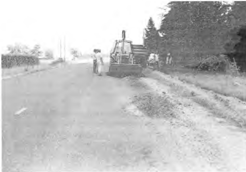
Figure 4. Patching one of the worst deteriorated areas before placing binder and surface.
