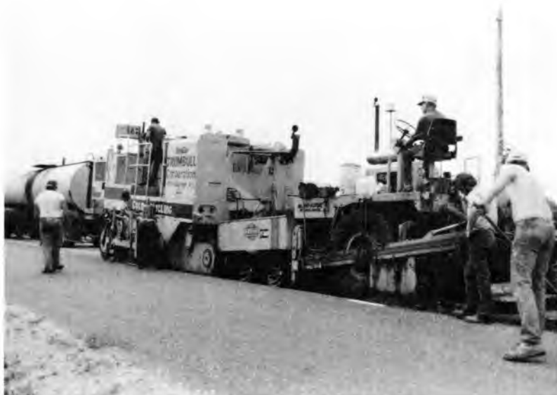
Figure 3. The supply trucks, recycling machine and paver work closely together in a recycling train.
