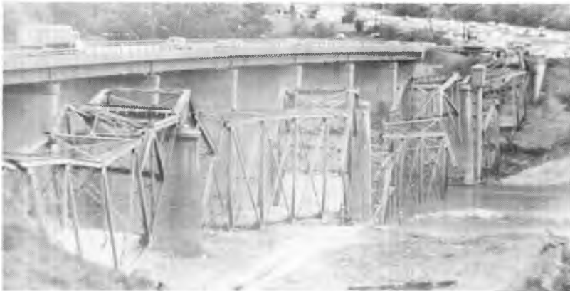
Figure 5. Final result of explosion.
