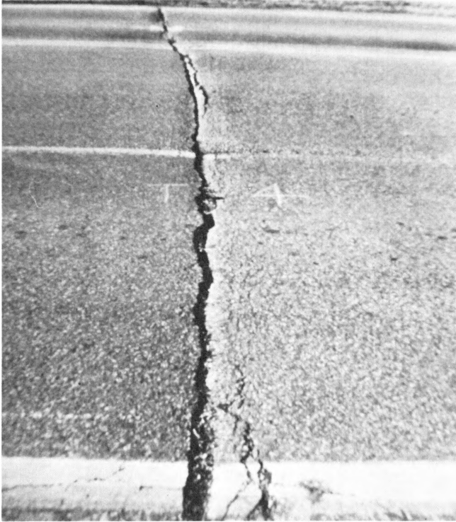
Figure 10. This is a typical Class 4 crack where the deterioration has progressed dramatically from the Class 3 crack. There is no evidence of maintenance repair procedures.
