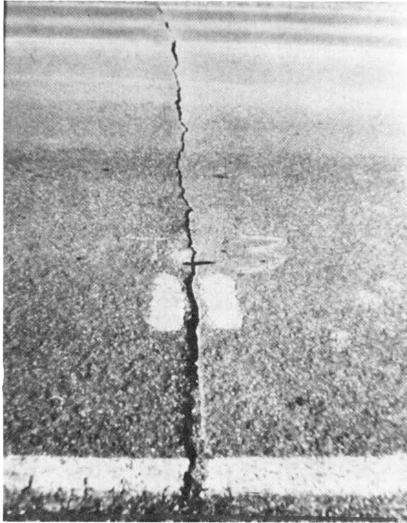
Figure 8. This typical Class 3 crack on the U.S. 71 project had no prior crack sealing or maintenance treatment. The classification of this crack is made by a 1/2-to 1-in. average depression. It is nearly a straight line transverse crack and occasionally a secondary crack develops on either side of the primary crack.
