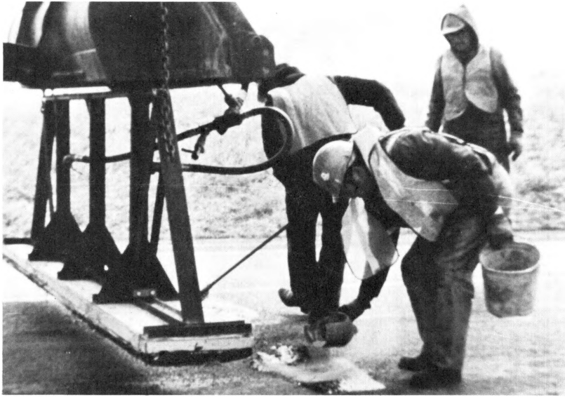
Figure 34. After strike-off of the crack, it was lightly dusted with a fly ash. The fly ash was available because our early inclinations were to use fly ash rather than limestone for the slurry mixture. We found that it did not have the desirable mix characteristics that we found in the limestone-slurry mixture.
