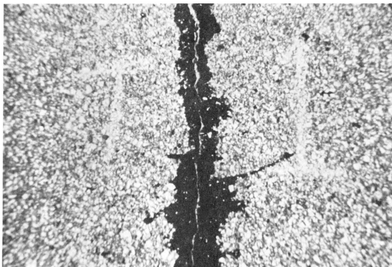
Figure 3. A closeup of that same Class 1 crack with the typical surface crack sealing that had been practiced universally over the state for many years.
