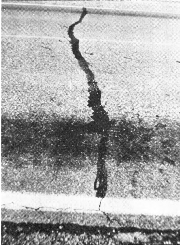
Figure 5. A typical Class 2 crack with maintenance crack filling treatment.
