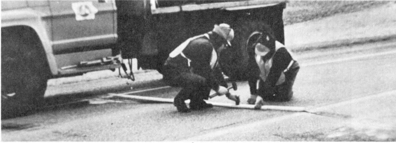
Figure 23. We believe the best time of year to fill asphalt pavement cracks is in the coldest part of the winter or early spring when the cracks are at their maximum opening. This slide shows a two-hole template to mark the positions on the pavement where the nozzles of the pressure truss applicator would be positioned. Only two nozzles are provided on the truss to accommodate positioning along an irregular transverse crack. After the locations were positioned with the template, a hydraulic jack-hammer driven by the maintenance truck's hydraulic system was used to drill the pilot hole for the pressure filling operation.
