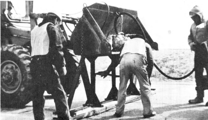
Figure 31. The pressure of the air reservoir of the compressor is applied to the pneumatic pump. We found that usually a 60 psi pressure on the pump was more than sufficient to pressure inject the slurry into the cracks. We would continue pumping until the slurry material started to extrude at the end of the platform section. In one instance where a crack had seriously faulted and the pavement sagged adjacent to it, we applied the full 120 psi to the system. We were slab pumping the pavement and actually lifting the depressed asphalt pavement back up to its original constructed elevation. This did not necessarily work in all situations because it depends on the configuration of the cavity beneath the crack.
