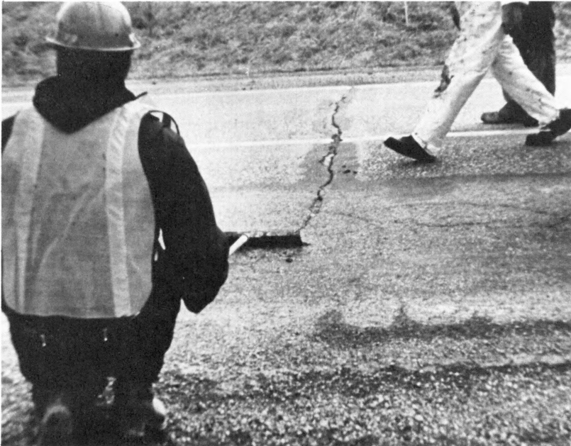
Figure 26. The crack sealing operation described here was limited largely to the Class 3 and Class 4 cracks, of which there were more than 3,500.
