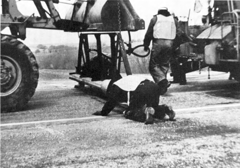
Figure 27. This typical Class 3 crack is being prepared for filling. The truss section was simply suspended under the loader bucket with a log chain in order to make the truss easily positioned as it was centered over the nozzle pilot holes. It then was lowered into position with the loader bucket.
