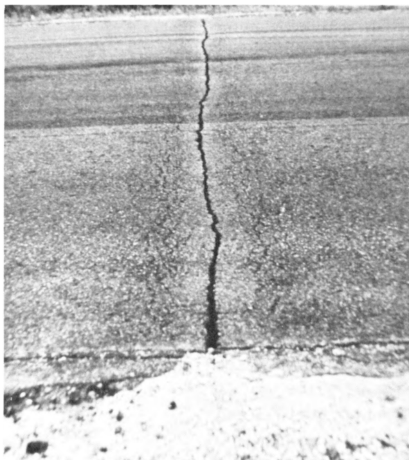
Figure 1. A closeup of a typical thermal crack on a rural asphalt pavement. Note in the close foreground that the fines of the granular base material are actually pumping out of the pavement onto the shoulder, causing an undermining of the pavement slab and the depression along the crack manifested in alligator cracking.
