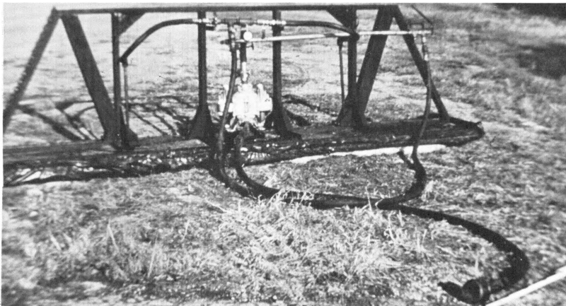
Figure 15. In order to accomplish this, we built this steel truss section that is approximately 11.5 ft. long. The platform is about 18 in. wide, is covered with a 2-in. solid plank platform which is further covered with a 3-in. mat of high density, flexible polyurethane foam covered by a polyethelene membrane. A pneumatic pump is mounted in the center of the truss section and to it's right and left about 4 ft. is the extension of nozzles that protrude through the bottom of this platform. In the foreground, a suction hose sucks slurry into the pump and through the nozzles into the pavement cracks.
