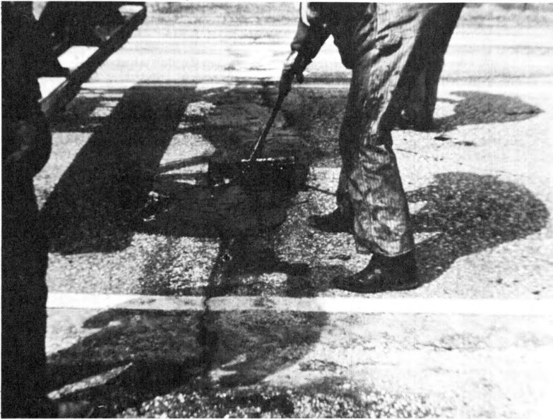
Figure 33. In areas where there was a transverse trough depression along the axis of the thermal crack, this trough was squeegeed full with the pressure injection slurry material. Note a wet spot in the foreground in the shoulder area adjacent to the crack. We found it not uncommon to pump from 7 to 15 gal. of slurry mixture into some of these cracks. In a few minutes a 6- to 10-ft. diameter circular area saturated with moisture would develop on the shoulder which indicated that the pressure slurry material was displacing the water in the cavity of the crack and was filling and waterproofing this area.
