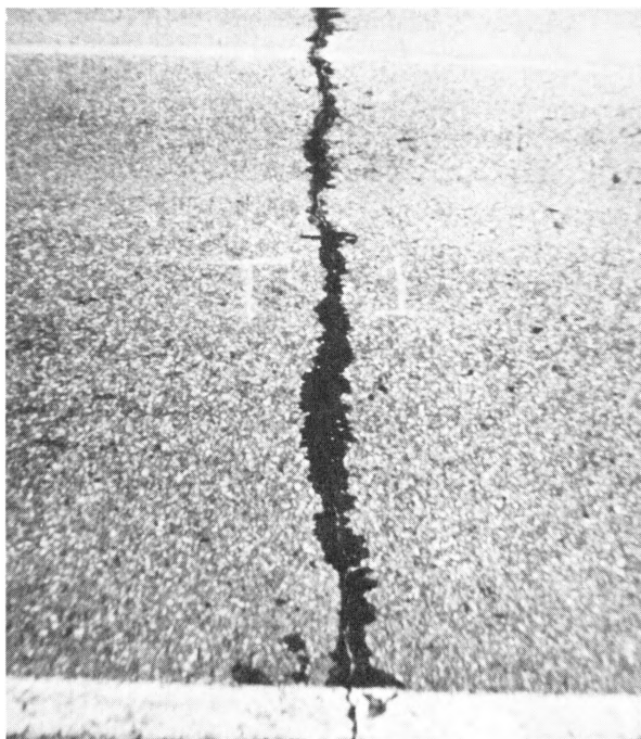
Figure 2. In an earlier analysis of our typical thermal cracks on the Iowa asphalt pavement sections, we have classified cracks into four categories. This is a typical Class 1 crack on a rural asphalt pavement.
