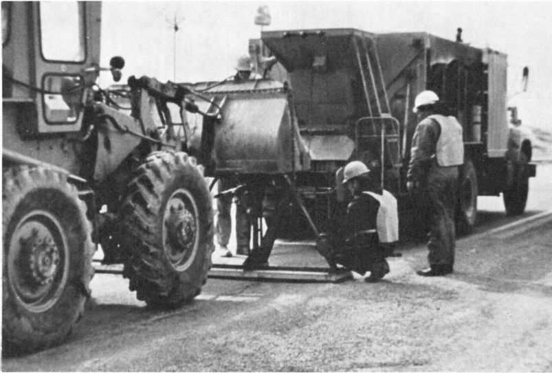
Figure 28. The total down pressure of the loader and its bucket was applied to the truss section. This pressure would compress the high density foam on the underside of the platform which would actually seal off the pavement surface at the crack interface so that high pressures could be applied and slurry injected into the cavities in the lower elevations of the pavement.
