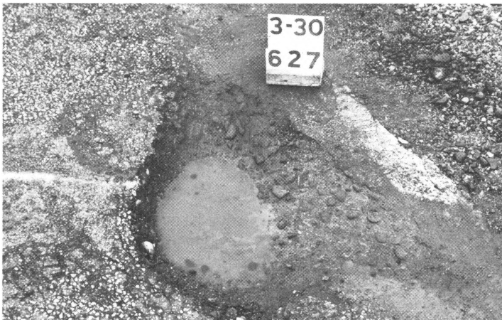
Figure 7. Typical Potholes on U.S. 52.
