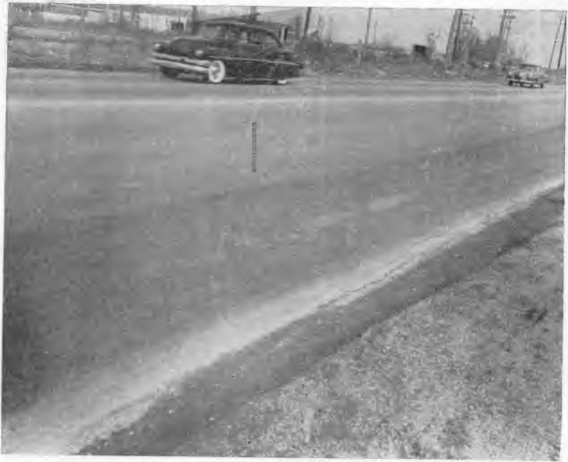
Fig. 6. Concrete exposed by rutting.
