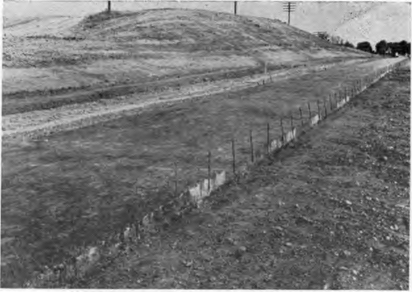
Fig. 2. Installation of tie bars across center line joint presented a problem with first machine.
