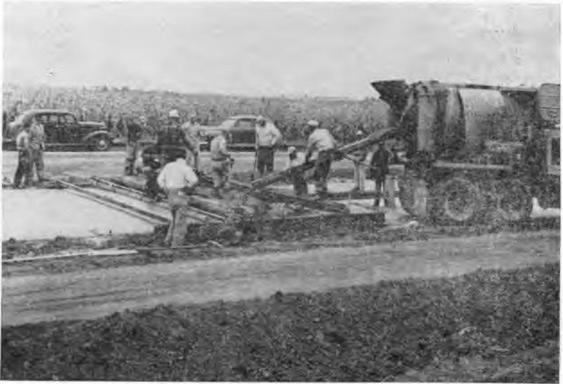
Fig. 3. Second machine developed. This unit was designed to construct a 22-foot course.
