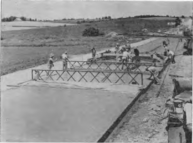
Fig. 7. Second self-propelled machine incorporated a permanent 22-foot slip-form and a temporary 16-foot slip-form, making a total length of 38 feet.
