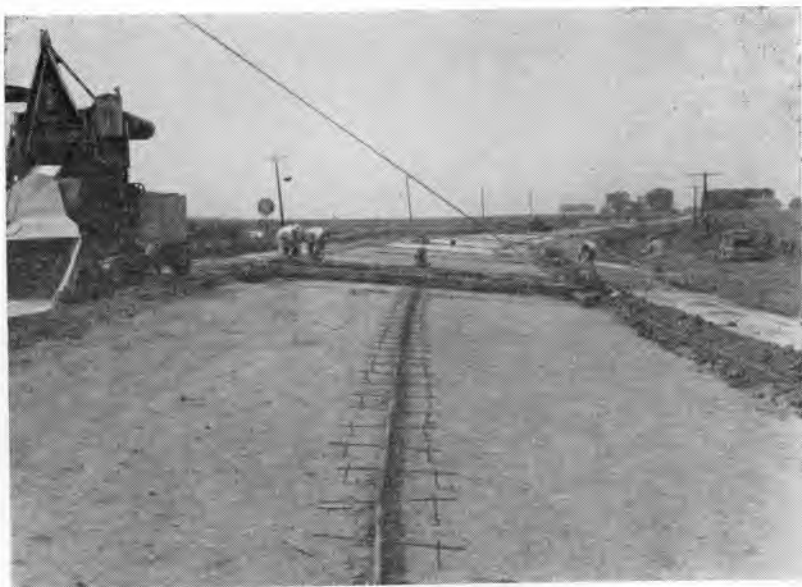
Fig. 4. A third machine was designed to construct a full-width course on super-elevated curves.
