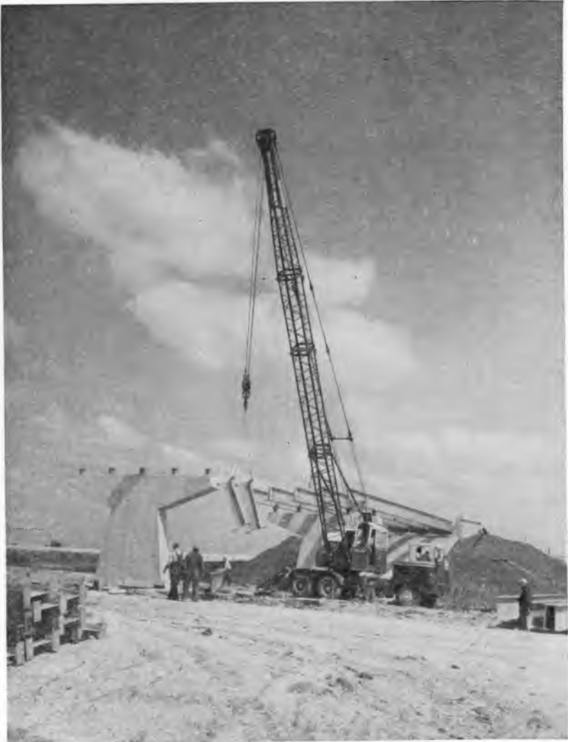
Fig. 3. Four overpasses carry local roads across the main test loops at the AASHO Road Test. When testing is completed, the main loops will be rehabilitated to become part of US Route 6 in the interstate highway system.
