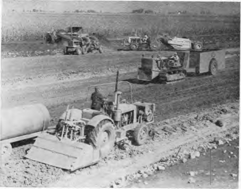
Fig. 2. Four types of equipment played major roles in the grading phase of the AASHO Road Test construction. Shown here are a rotary speed mixer (foreground), a pneumatic compactor (right center), and a blade grader and two earth movers (background).
