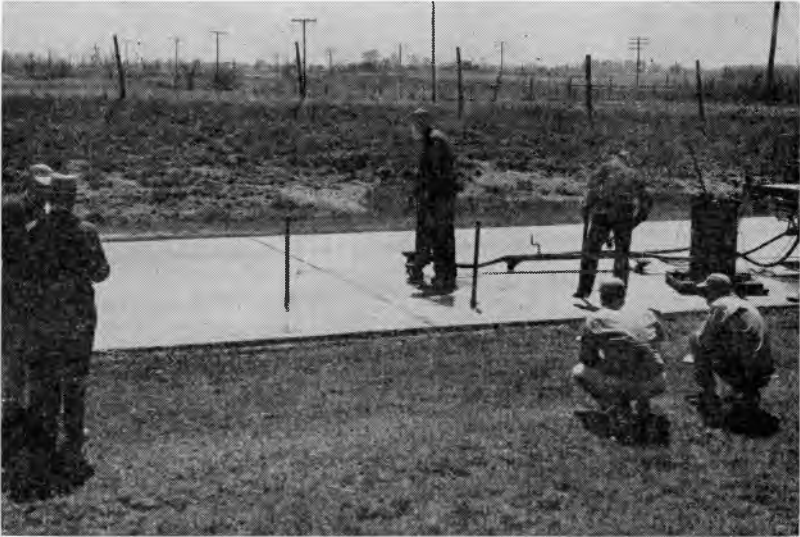
Fig. 17. Crew undersealing pumping pavements with extremely hot bituminous material. This maintenance operation has made possible the salvage of many miles of high-type pavement in Indiana. (18839)
