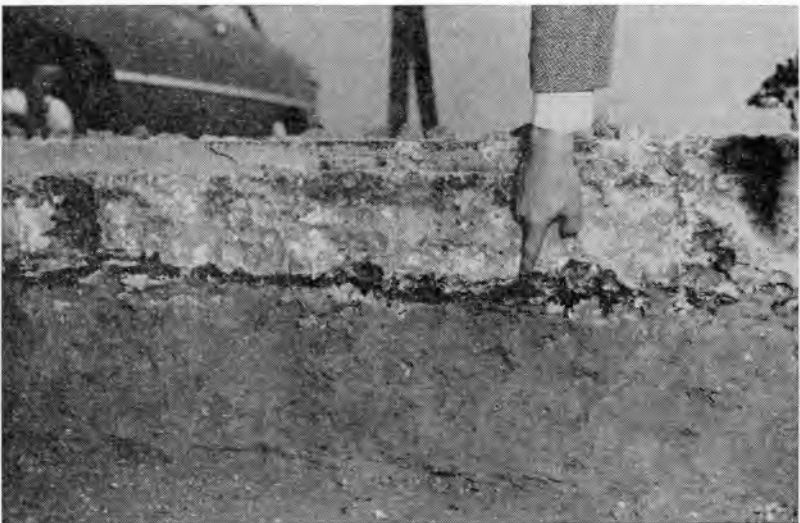
Fig. 18. Undersealing placed under pumping pavements. Note bituminous material under rigid pavement. This maintenance operation has proven quite successful in retarding the pumping out of subgrade soils from beneath rigid pavements. (18333)
