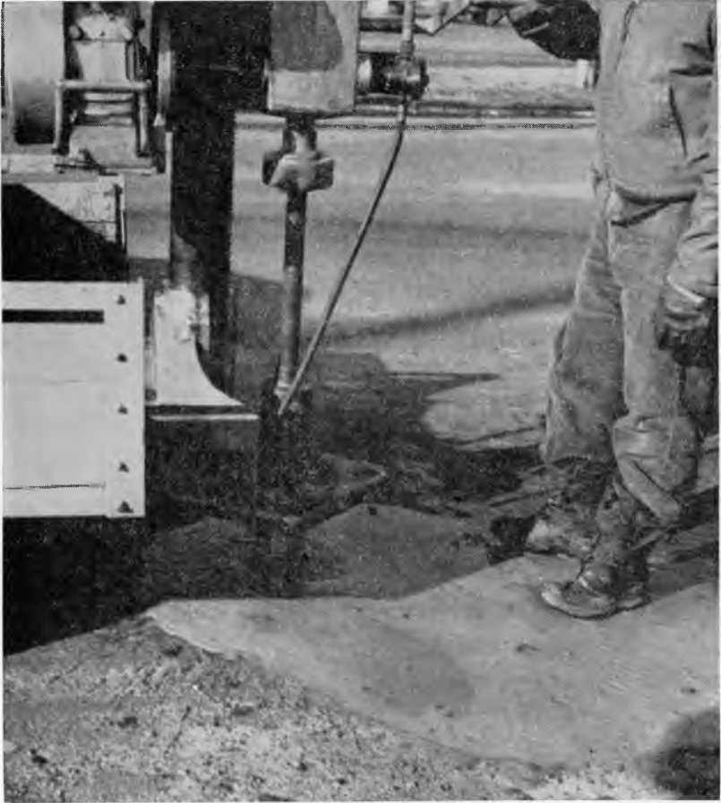
Fig. 8. This view shows one method of obtaining cores of bituminous concrete resurfacing for laboratory tests. (34787)
