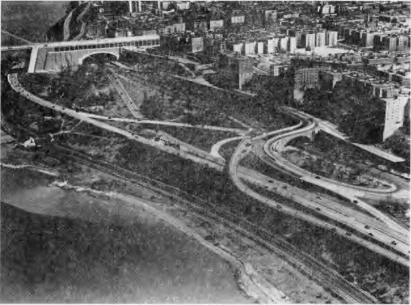
Fig. 2. New exit ramp under construction (foreground) will connect George Washington Bridge with Henry Hudson Parkway, eliminating present circuitous route and traffic grade crossing.
