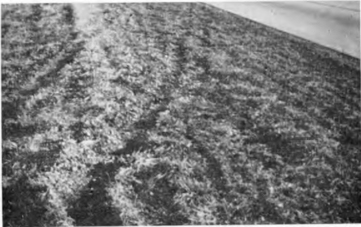
Fig. 13. View of granular stabilized shoulders. Note the deep ruts cut into the natural subgrade and lack of driver control on the soil.
