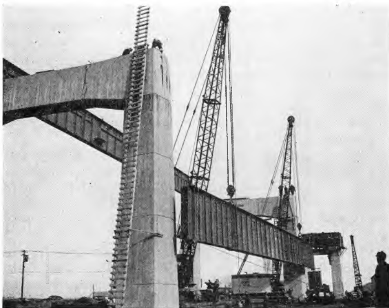
Figure 1. Steel girders being placed on concrete piers at the Passaic River Crossing.
