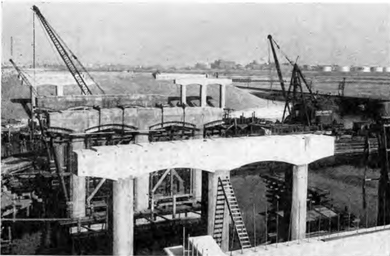
Figure 3. Construction of substructures for the Rahway River crossing. This dual crossing provides two separate parallel structures, one for northbound traffic and the other for southbound traffic. Both will be identical in size and design.
