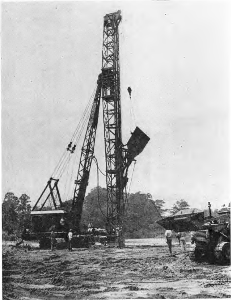
Figure 4. Placing "sand drains" up to 100 feet in depth through swampy areas has speeded up the consolidation of road embankments. This figure illustrates one type of rig used to install sand drains.
