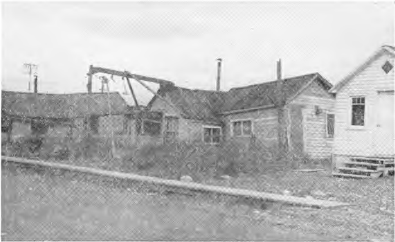
FIGURE 7. Severe settlement of a house resulting from thawing subsoils.
