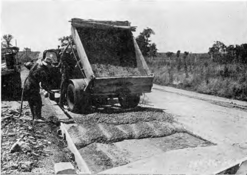
Concrete replacement using wet-batch method. Note use of vibrator to insure better joint between old and new concrete.
