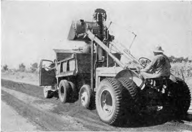
* Loading mixed material for hauling to point of use—either for decking or patching.
