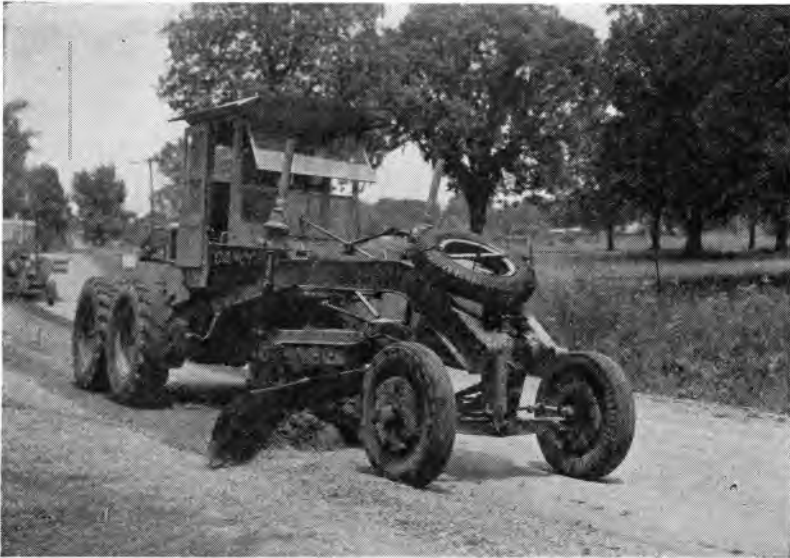
Gravel road maintenance. Note use of motor graders working in tandem. Best results are accomplished by this method.
