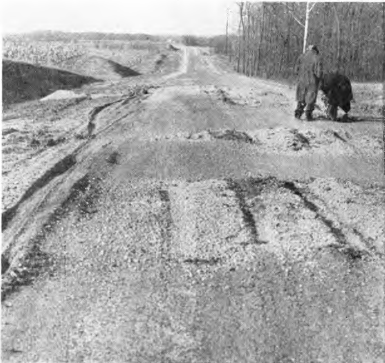
Fig. 2. Typical failure of a secondary road where the grade line cuts into parent material—rolling topography of the Wisconsin-drift area.
