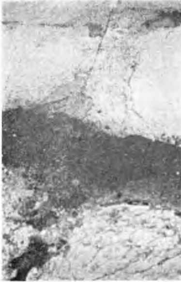
Fig. 7. Typical example of severe map cracking associated with a blowup.
