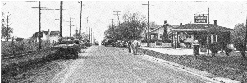
Fig. 1. Widening with concrete along brick section of U. S. Highway 31 at Whiteland preparatory to resurfacing.
