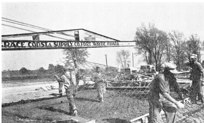
Fig. 2. Steel mesh reinforcing no longer used in construction because of war priorities.
