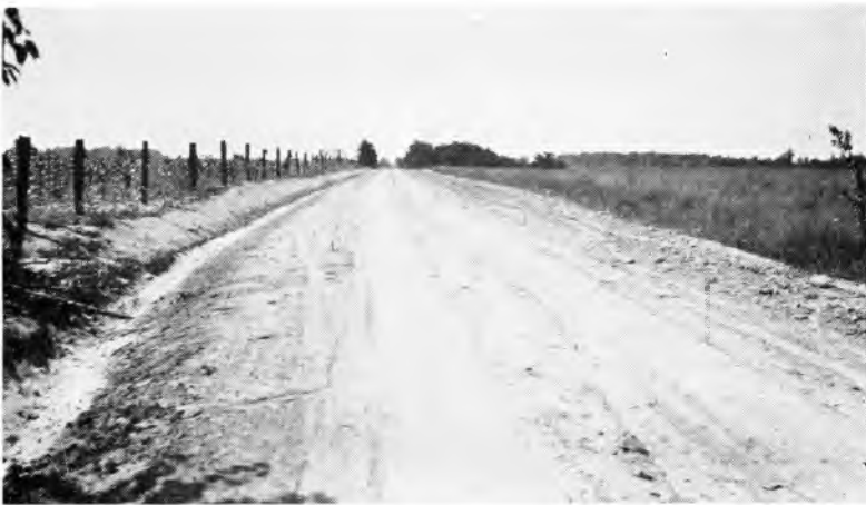
Fig. 2. A typical graded and drained section of earth road ready for crushed stone surfacing in Ripley County.
