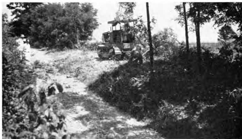
Fig. 1. Clearing and grubbing preparatory to grading, draining, and surfacing an unimproved earth road in Ripley County.
