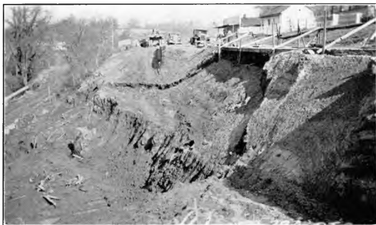
Fig. 1. Embankment failure after a severe flood, Washington County.
