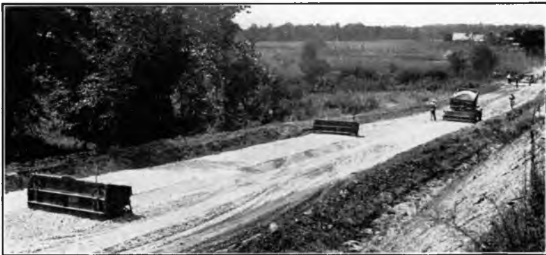
Fig. 3. A stabilization project on the Spencer-Ashboro Road in Indiana, illustrating method of placing plant-mixed materials by means of trucks and spreader boxes.
