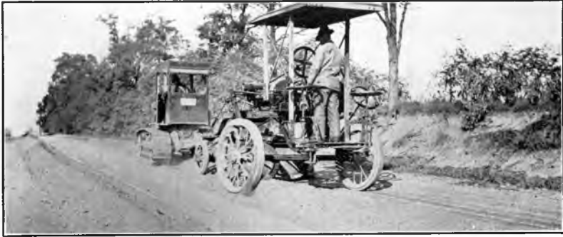
Fig. 2. A stabilization project in Washtenaw County, Michigan, illustrating mixed-in-place operations using a tractor and a road grader.
