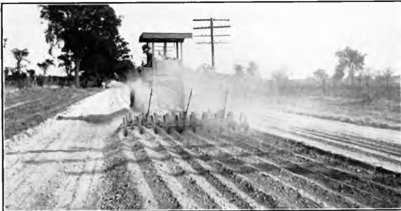
Fig. 1. A stabilization project in Lenawee County, Michigan, illustrating mixed-in-place operations using a tractor and a spring-tooth drag.
