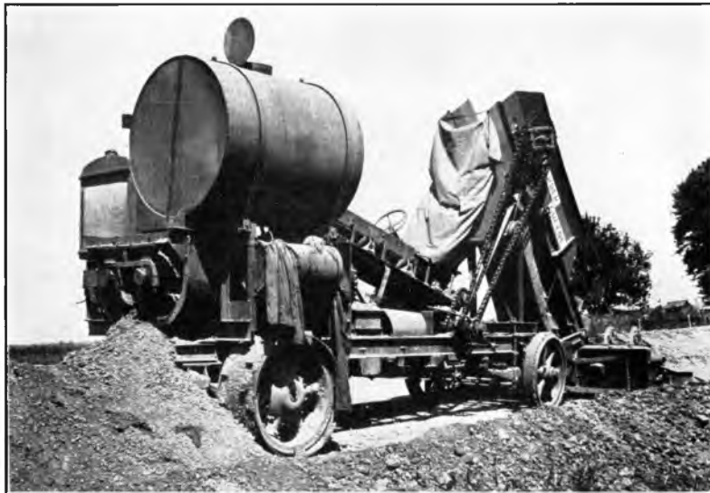
Fig. 5. Wapella project in Illinois illustrating use of Barber Greene road mixing machine in stabilization work.
