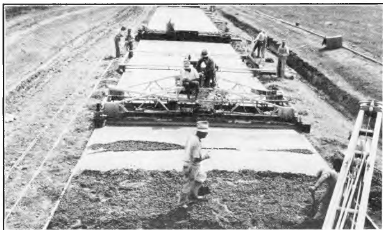
Fig. 5. Vibratory finishing machine used in experimental construction. Note man walking on top of mixture.
