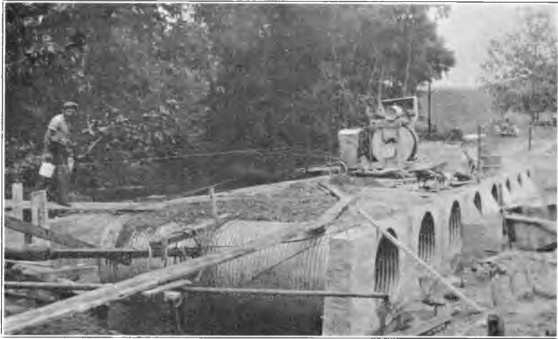
Fig. 4. Pipes in place. Note butresses between pipes to aid in passing debris.
